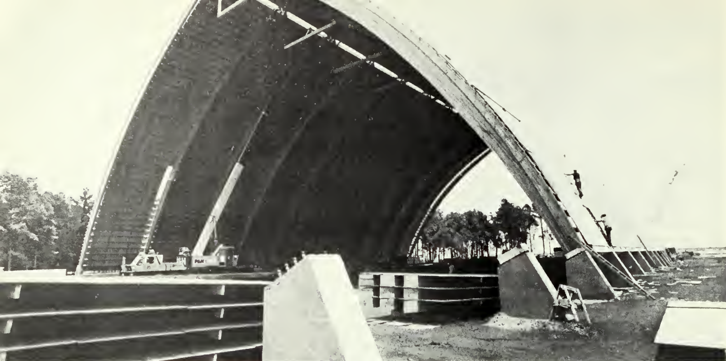
Giant export facility warehouse is shown under construction on Colonel's Island. Now completed and operational, the new warehouse was built entirely of Southern yellow pine. Architectural designers determined concrete and steel were unsuitable for construction because of highly corrosive materials to be stored. The pine structure, treated with fire retardant chemicals, is expected to last indefinitely.
