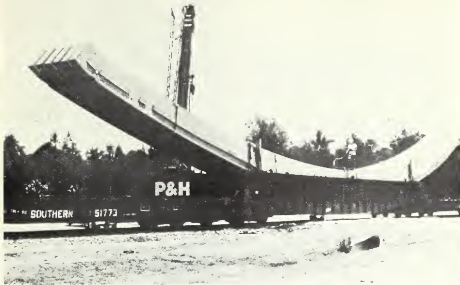
Specially designed 127-foot-long roof members are transported to Colonel's Island by flat-bed railroad cars during warehouse construction. Adhesives, stronger than wood, were used to form the one-piece laminations which were tested for load capacity and cured to exact curve designated by architectural plans.
