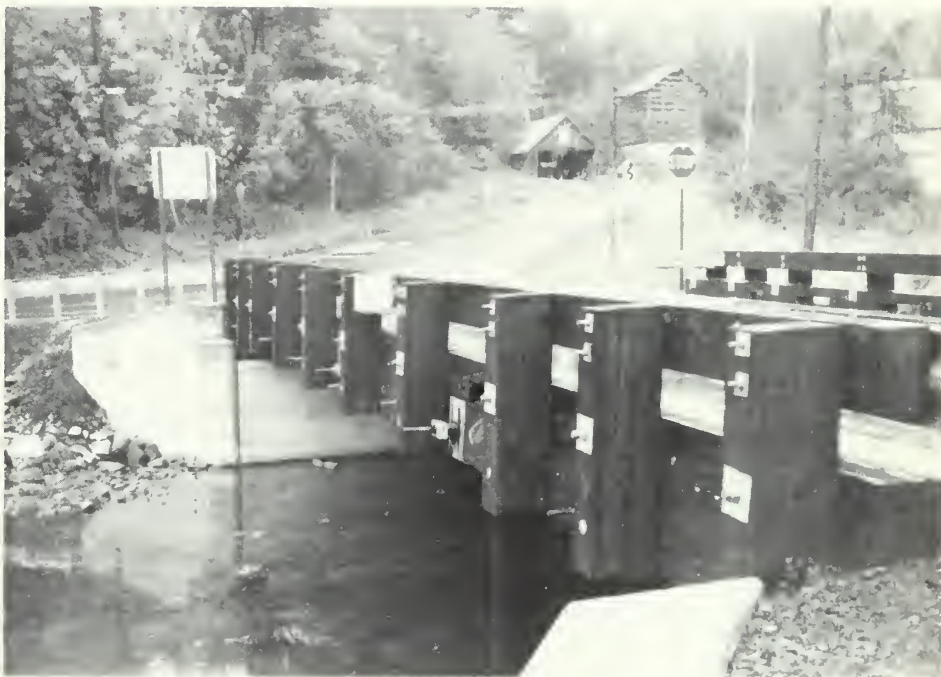
This bridge of pressure treated softwood prefabricated panels was assembled on the abutments in just one day. The bridge, located in a rural section of Pennsylvania, is typical of the type span the Georgia Forestry Commission is advocating for replacement of some old bridges in Georgia.
