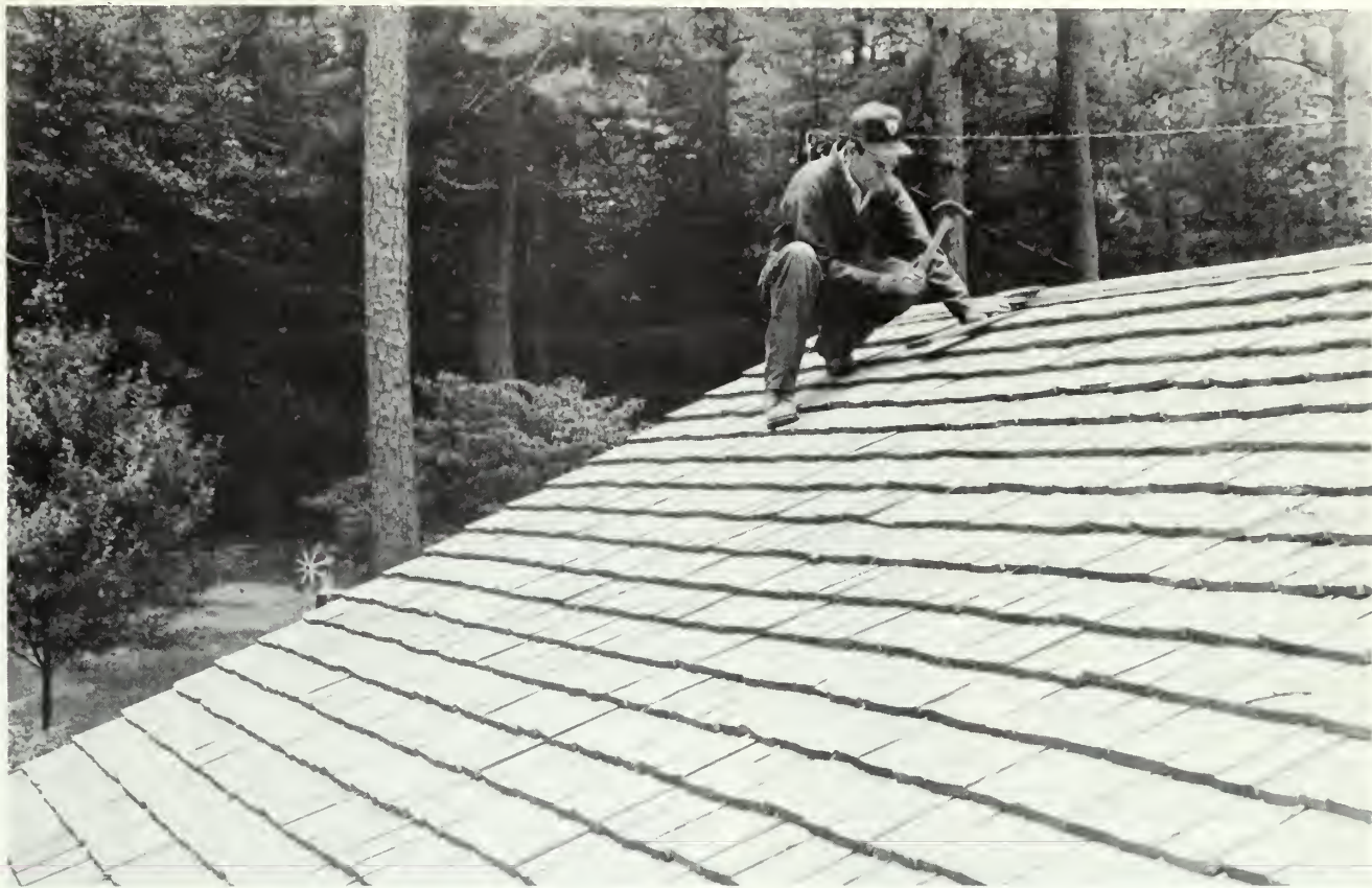
Patrolman Randy Sockwell replaces a shingle on the roof of the commission's Urban Forestry headquarters at Stone Mountain. The roof of chemically treated pine shingles is one of several unique features of the building which is visited frequently by builders and others interested in innovative uses of wood. The structure is built on a treated all-wood foundation. The building is one of several new commission offices that are roofed with shingles manufactured from Georgia pine.
