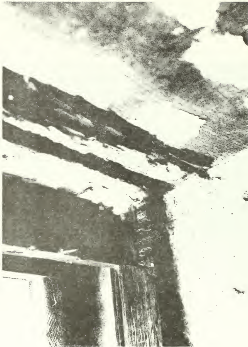
14. Deteriorated lintel in a west nave window.
