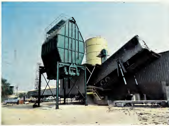
The fine sawdust is stored in a newly constructed silo with built-in safety devices against explosion.
