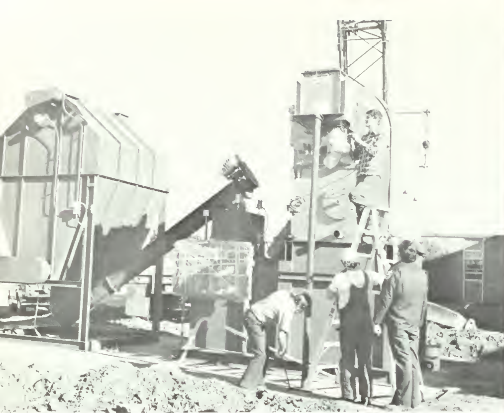
Workmen install heating equipment for Franklin County school. A building was later constructed around the installation.
