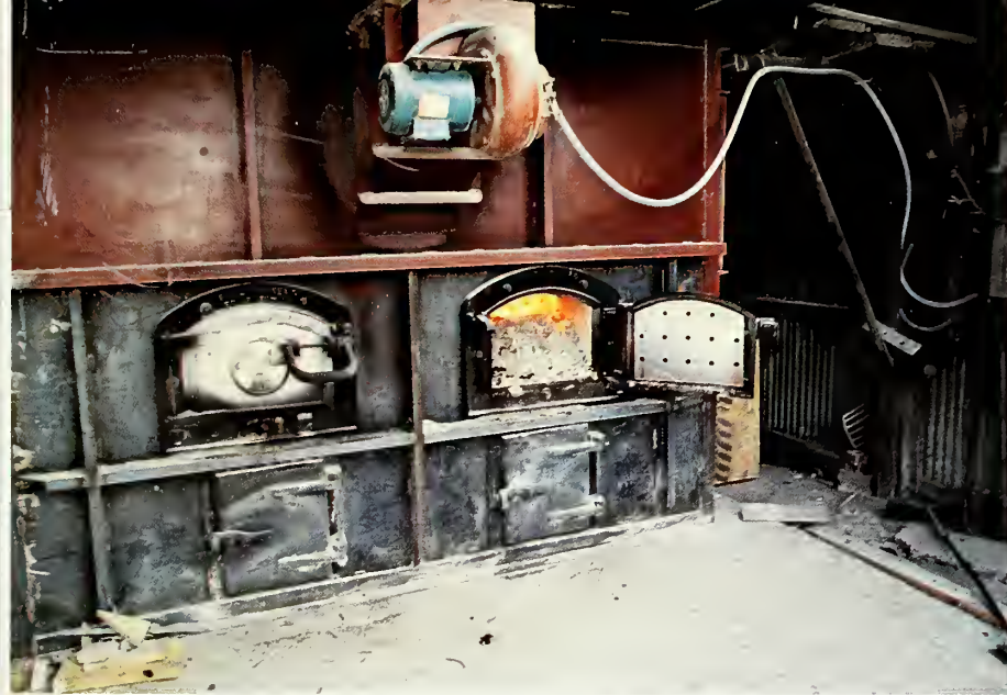
A modern wood-fired boiler produces steam for a sawmill operation.
