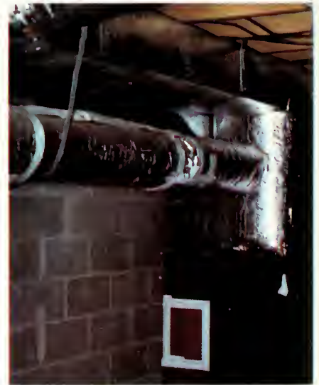
The wood furnace of Joe McCoy requires about 4-5 sticks of wood four times per day. Hot air ducts carry heat from the fireplace to each room in his north Georgia home.
