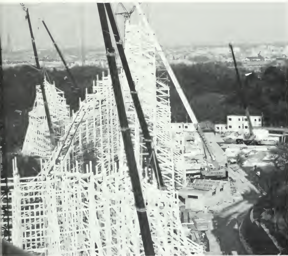
Japanese cranes set sections of giant wooden roller coaster in place. More than a billion feet of Georgia pine were shipped to Japan for this cyclone-style (figure 8) coaster.
