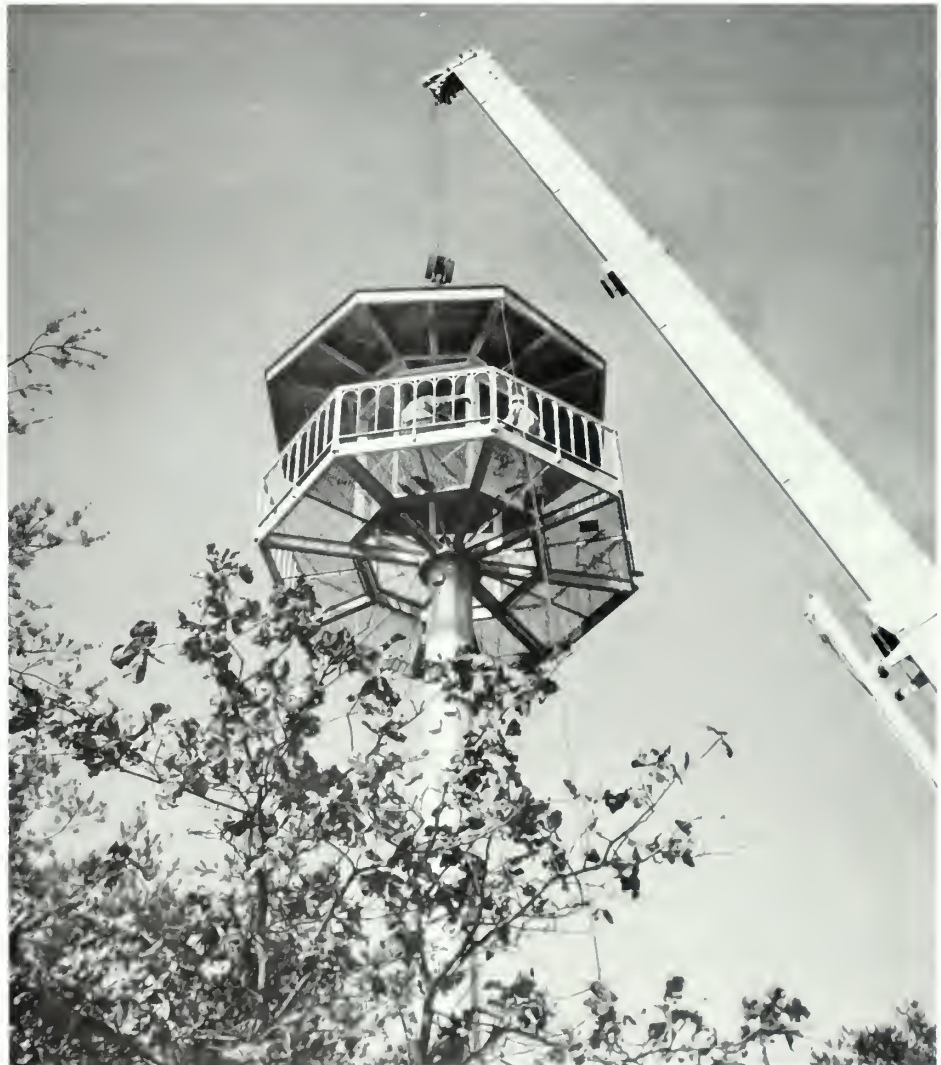
Construction crew works on structure that replaced the Commission's standard forest fire lookout tower on Sawnee Mountain.
