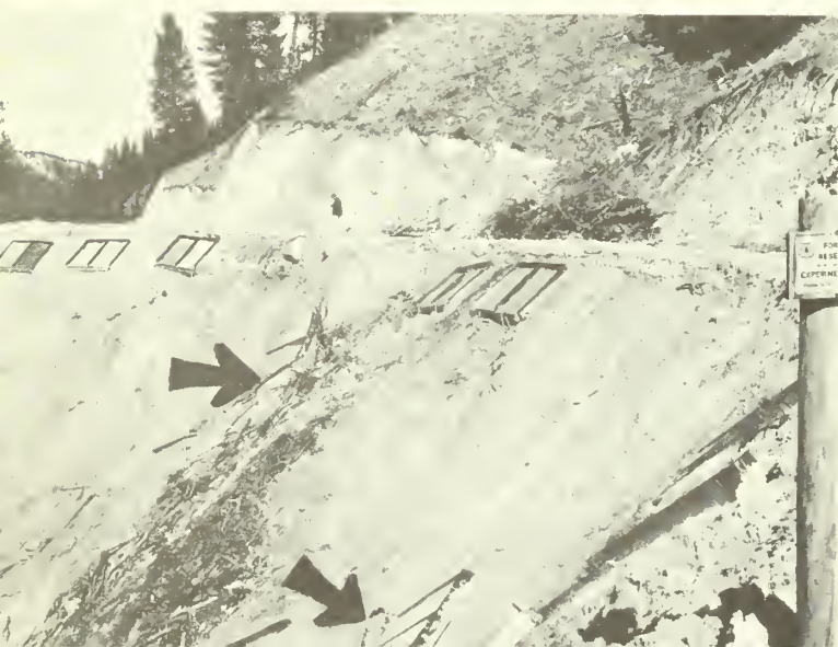
Figure 4.--Appearance of an insloped section of road set aside for plot studies following the October 1962 storms. Arrows locate plot frames displaced from original position on incurves. Other plot frames remain nearly intact on outcurves.
