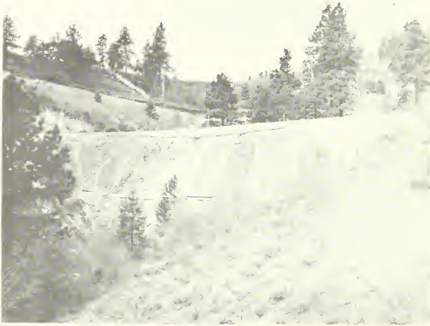
Figure 1. --Overall view of the test plots that were established on a steep fill slope on the Bogus Basin road.
