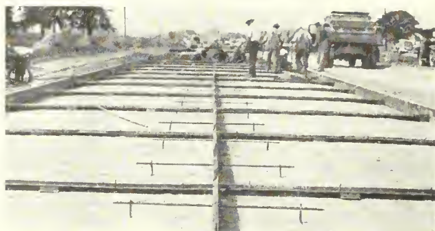
FIGURE 10.—DEVICES USED IN FORMING SUBMERGED WEAKENED-PLANE JOINTS IN PLACE ON THE SUBGRADE.
