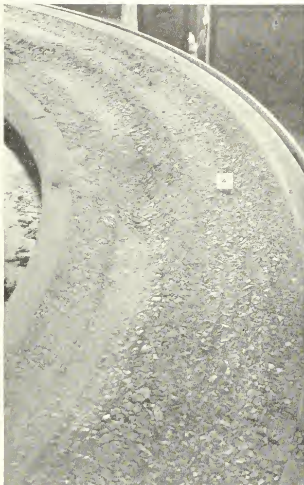
FIGURE 9.—APPEARANCE OF SECTION 4 OF SERIES 2 AT THE END OF THE TRAFFIC TEST (330,000 WHEEL-TRIPS). THE DEEP RUT IN THE INSIDE LANE INDICATED AN IMPENDING FAILURE.
