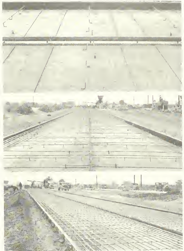
FIGURE 6.—INSTALLMENT OF HEAVY BAR REINFORCEMENT. TOP, WELDED CHAIR SUPPORTS AND TRANSVERSE BARS BEING PLACED; MIDDLE, LONGITUDINAL AND TRANSVERSE STEEL BEING PLACED; BOTTOM, HEAVY BAR MAT REINFORCEMENT IN PLACE.
