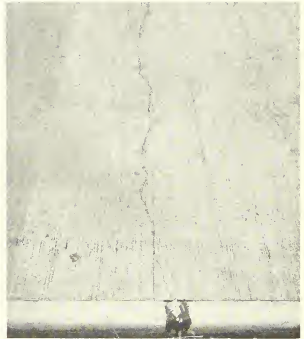
FIGURE 20.—TYPICAL CRACK IN A HEAVILY REINFORCED SECTION.
