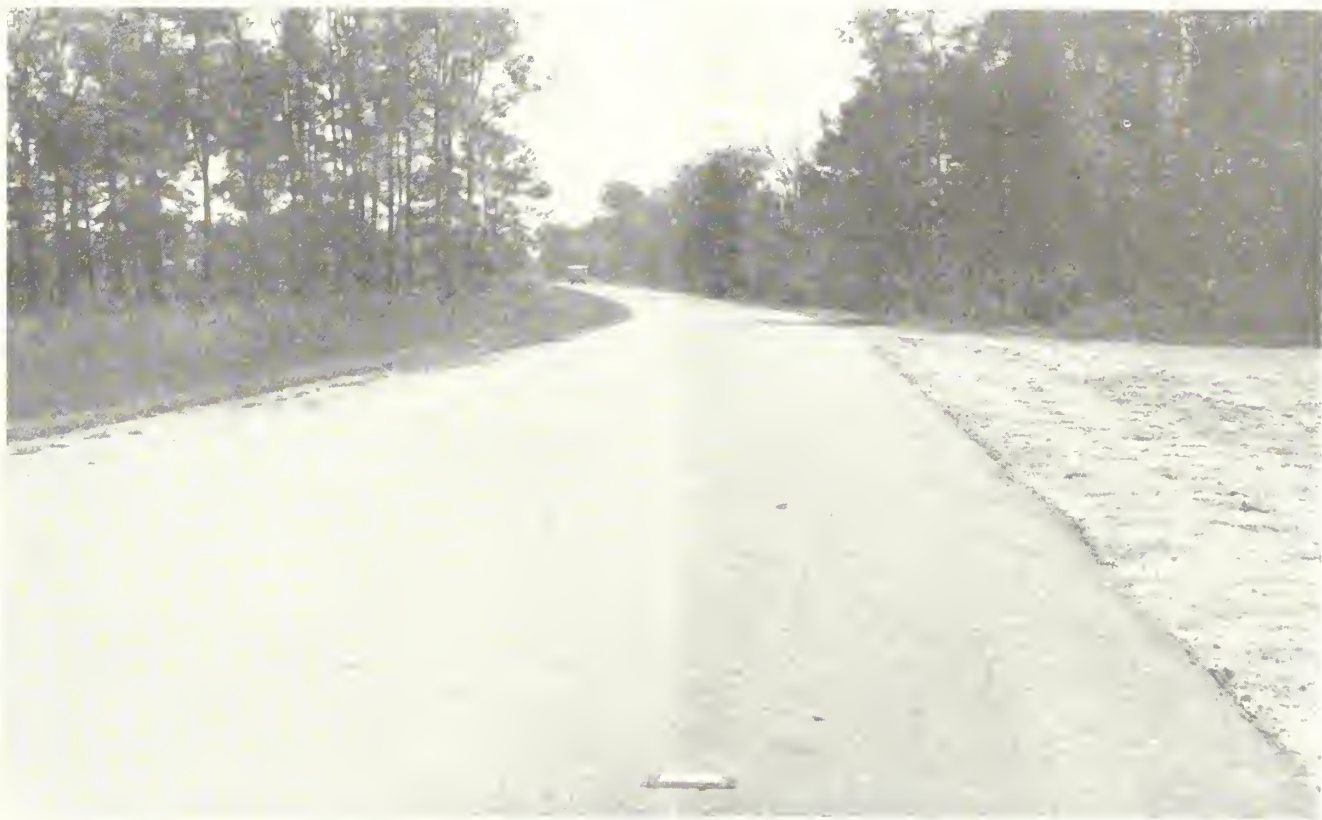
FIGURE 5.—GENERAL VIEW OF THE EAST PORTION OF EXPERIMENT 6A, WHICH IS TYPICAL OF THE ENTIRE SECTION. NOTE THE EVEN EDGES AND UNIFORM APPEARANCE.
