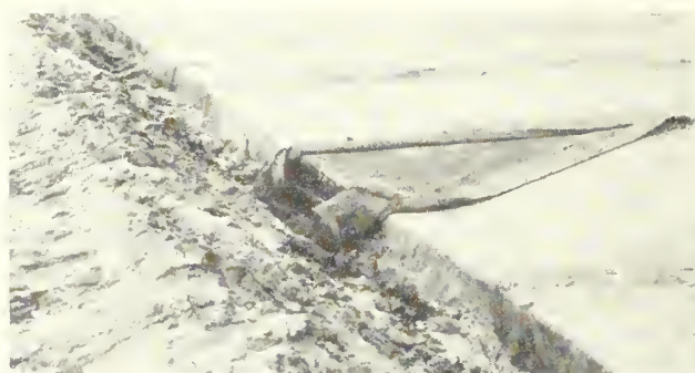
FIGURE 2.—COTTON MATS DISINTEGRATE RAPIDLY IF ALLOWED TO OVERHANG ONTO THE SUBGRADE AS SHOWN.
