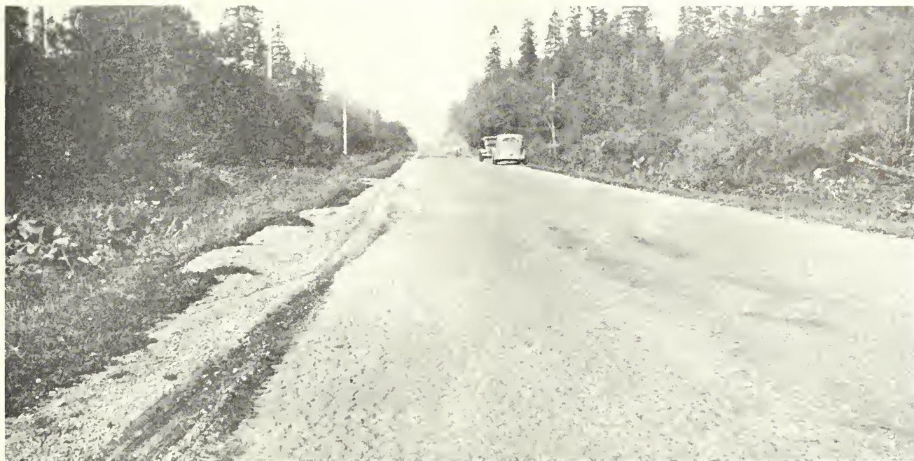
FIGURE 1.—EXISTING ROAD PRIOR TO RECONSTRUCTION. PICTURE TAKEN AT STATION 235, SHOWING CRACKS CAUSED BY UNSTABLE SUBGRADE.
