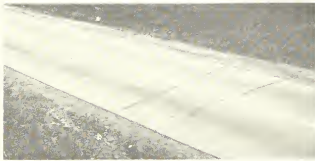
FIGURE 1.—PRESENT APPEARANCE OF A HEAVILY REINFORCED SECTION OF THE COLUMBIA PIKE EXPERIMENTAL PAVEMENT.
