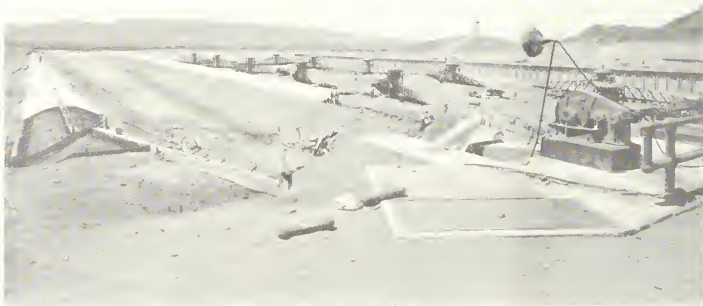
Bypass channel and effluent channel in foreground Rotary scrapers and influent channel in background
