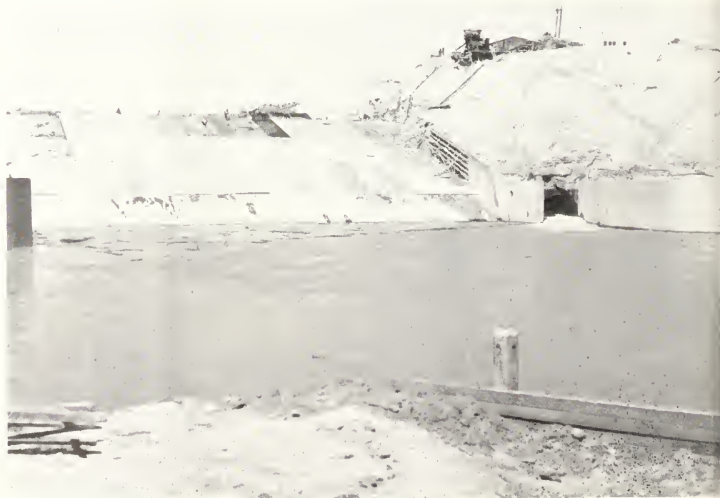
Fresno Dam from below spillway, showing water from tunnel after diversion, July 13, 1938
