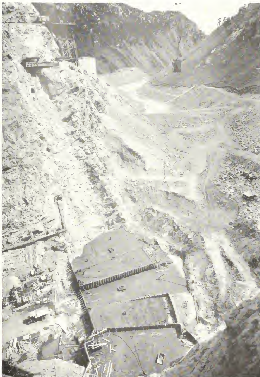
Seminoe Dam, Kendrick Project, Wyoming, the 260-foot structure being built by the Bureau of Reclamation, will block the North Platte River as it curves through steep Seminoe Canyon, 55 miles southwest of Casper, Wyoming. Note the dam appears to lie lengthwise of the river, as the sharp curve in back of the dam is now unwatered
