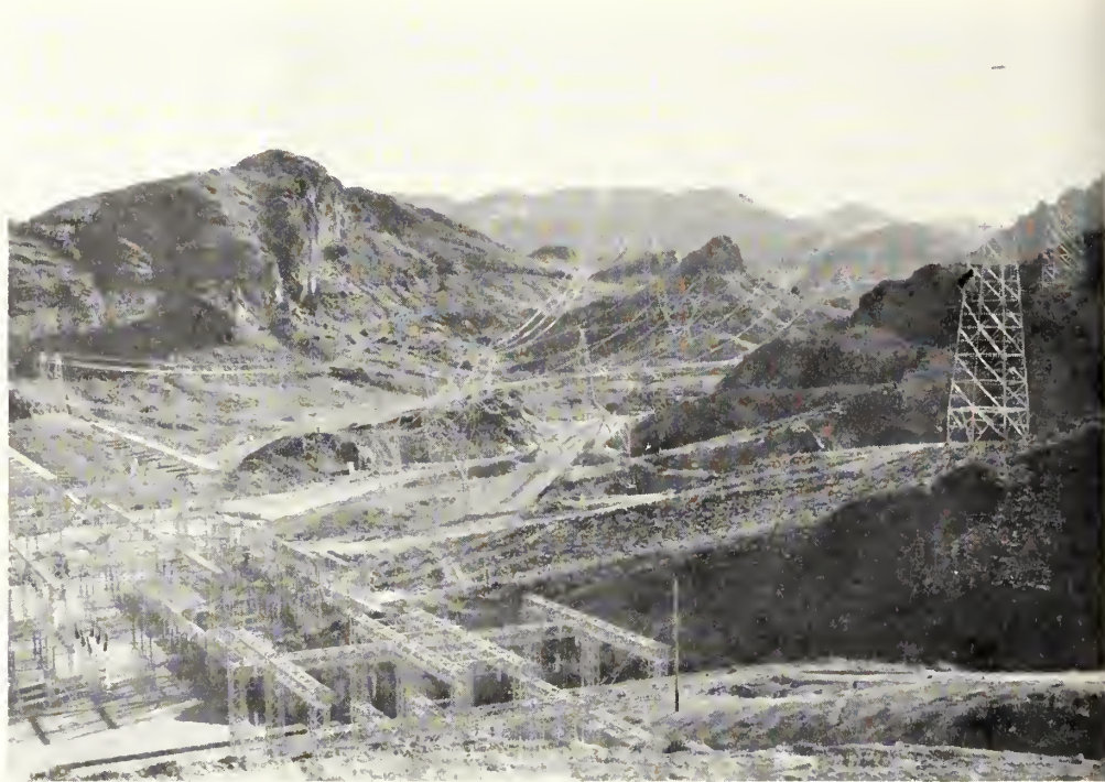
The City of Los Angeles and Nevada-California Electric Corporation switch yards and a portion of the transmission lines carrying power from Boulder power plant
