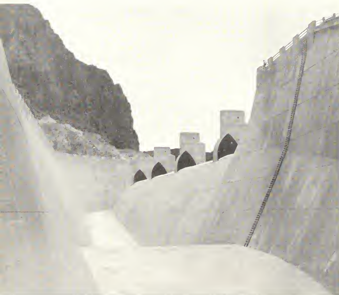
Spillways like these, one on the Arizona and one on the Nevada side, ready for overflow from Lake Mead
