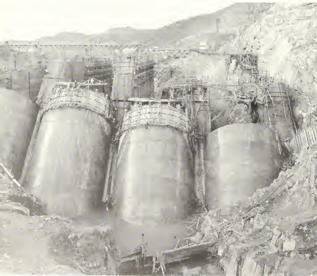
Top of arches are below river level
