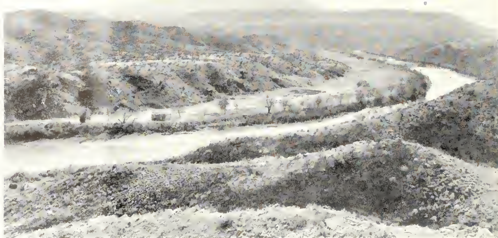
Site of fish hatchery being built by CCC on Rio Grande below Elephant Butte Reservoir.
