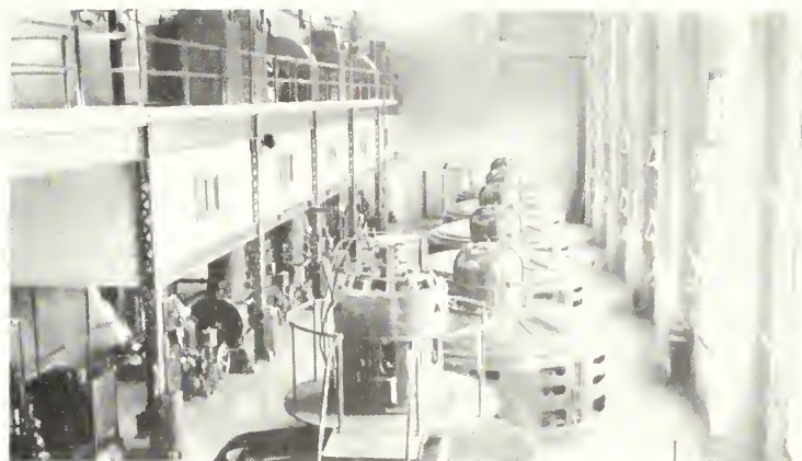
Minidoka Power House, generator floor
