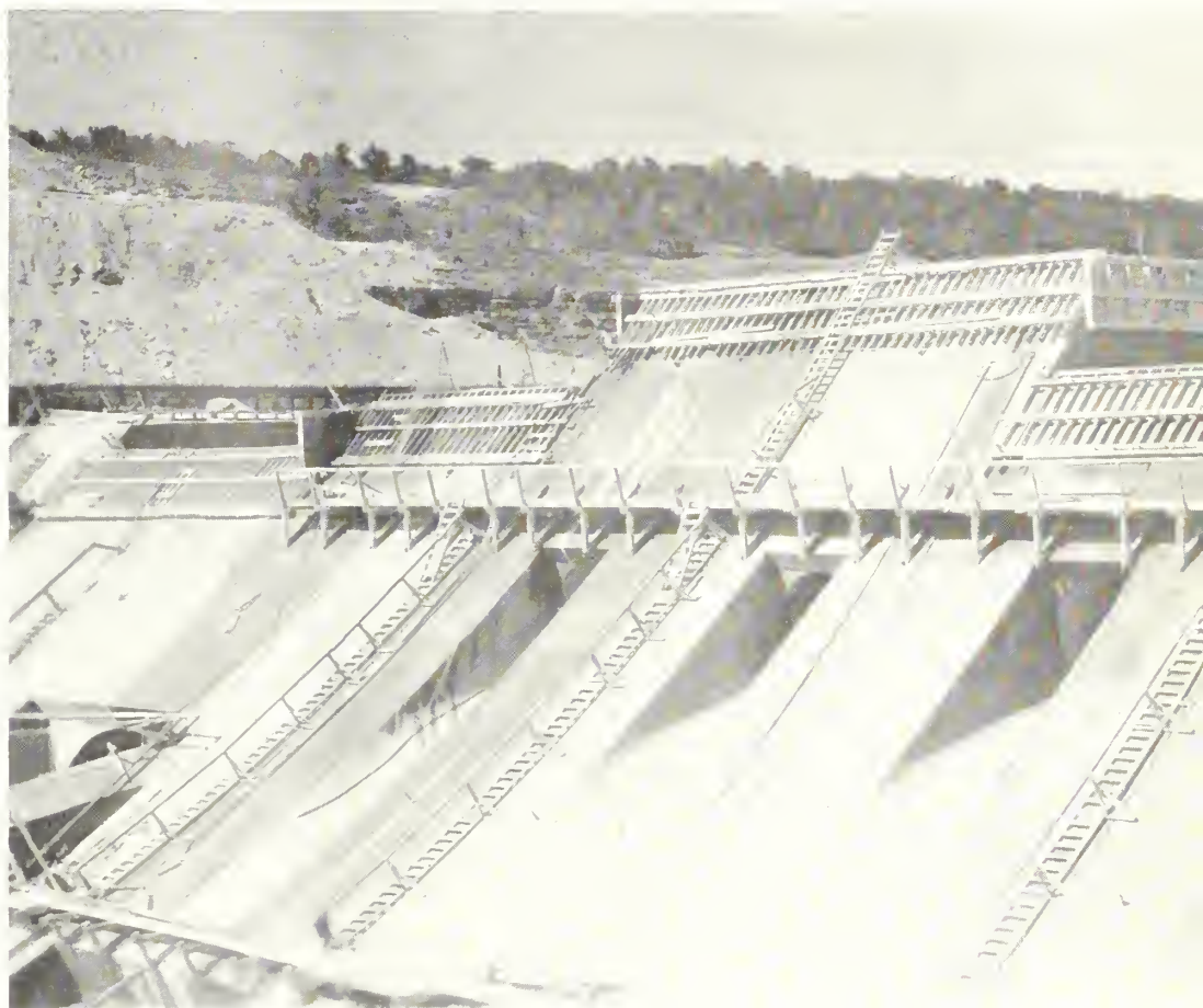
Downstream face of Parker Dam from California side of river; power-house substructure, initial construction, is complete in left foreground
