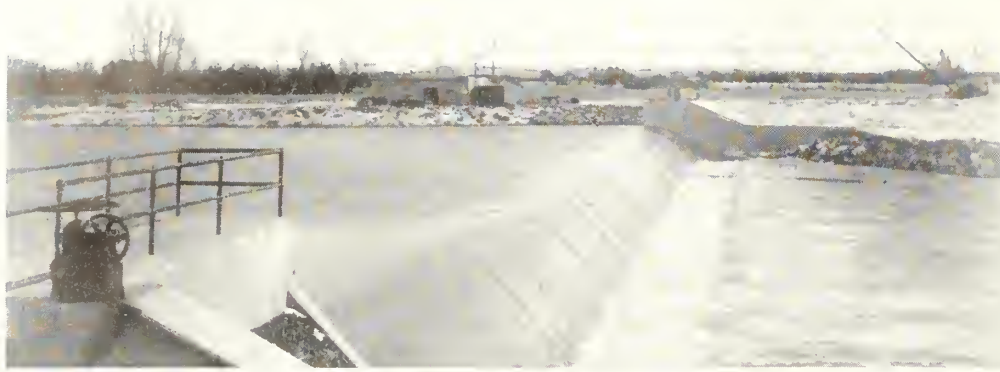
Cross Cut Diversion Dam from Last Chance canal headworks on right abutment. Note the effect of dentated sills at toe of dam. About 1,600 cubic feet per second is shown flowing over the dam
