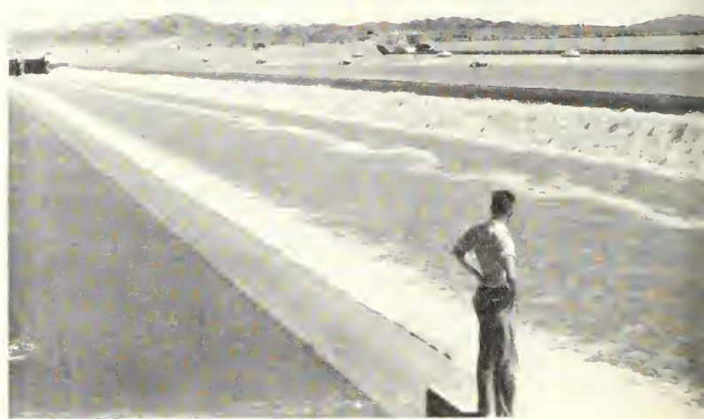
Clear water enters effluent channel
