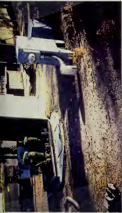
Typical example of a suction lift type pump station. This specific station is located at Katherine.
