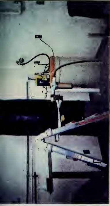
Typical polymer mixing and feed at water treatment plant.
