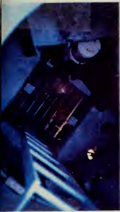
Typical access for flooded suction, package lift station.
