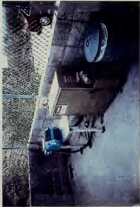
Roto-phase converter used to convert single phase power to three phase power.
