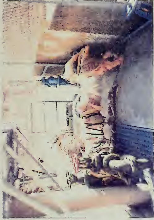
Insulated exterior water piping at Overton Beach.
