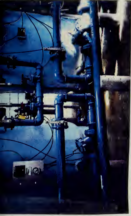
Pressure filters at Las Vegas Wash.
