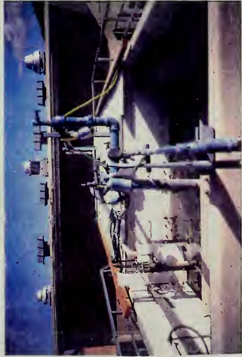
Typical package water treatment plant.
