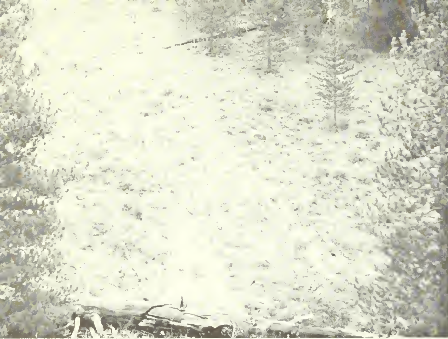
Figure 1.--Sediment dis- lodgment from an aban- doned logging road, Beaver Creek, Boise National Forest.
