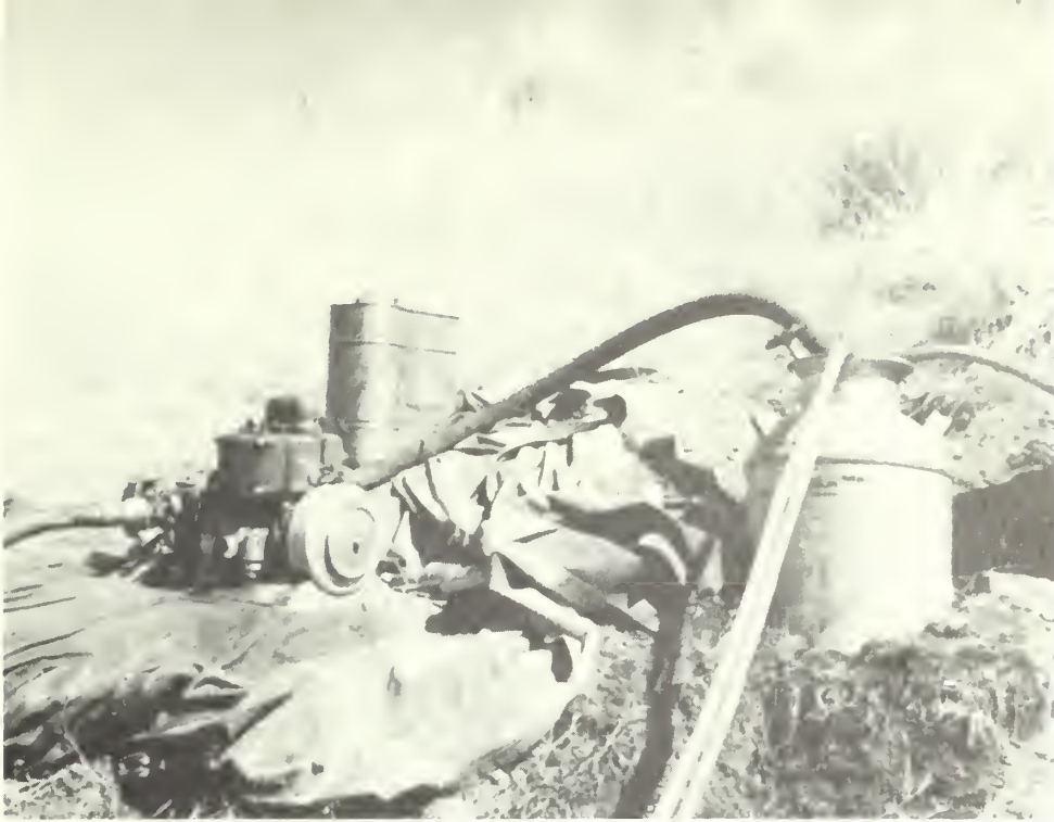
Figure 4.--Portion of pressure circulation unit showing the 10-gallon reservoir, suction hose, pump, and discharge hose.
