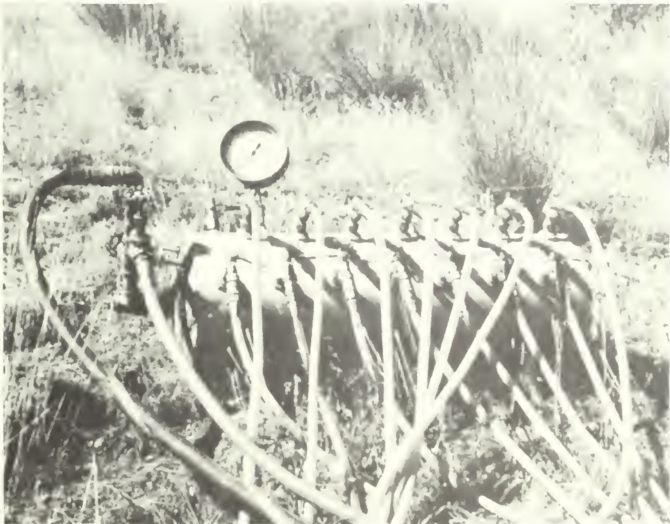
Figure 5.--Portion of pressure circulation unit showing pressure line from pump, pressure control valve, bypass valve, pressure control tank, relief valve, pressure gage, bypass hose, and 14 pressure lines to nozzles.
