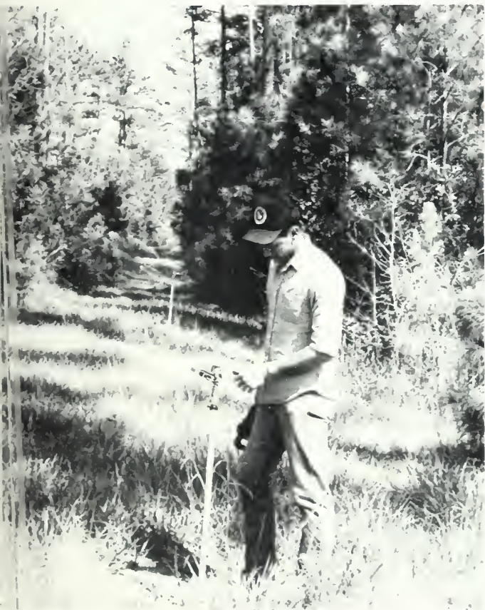
David Croom, manager of the Covington/Newton County Land Application facility, adjusts sprinkler on system that irrigates 550 acres of pine forests with domestic sewage. Pines absorb nutrients from the treated waste water that produces accelerated tree growth. Increased growth has been measured in pines ranging from seedlings to 100-year-old trees.
