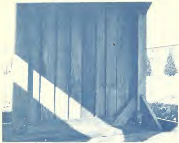
Figure 2.— Interior view of a shelter with board-and-batten siding. Boards are spaced \frac{3}{4} inch for expansion and shrinkage.
