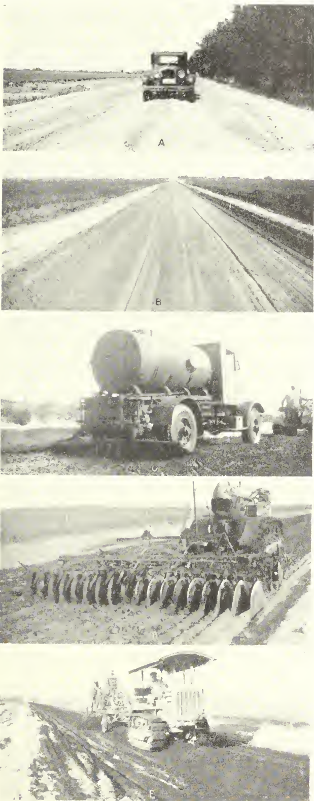
FIGURE 1.—APPEARANCE OF THE ROAD BEFORE AND DURING CONSTRUCTION OF THE BITUMINOUS SURFACE. A, PORTION OF SECTION 3A BEFORE BITUMINOUS TREATMENT. B, SAND FOR THE TOP 2 INCHES WINDROWED AT THE SIDES. C, BITUMINOUS MATERIAL BEING APPLIED AT THE RATE OF 1/2 GALLON PER SQUARE YARD. D, PRE-MIXING OF SAND AND BITUMEN WITH A DISK HARROW. E, UNIFORM MIXING WAS DIFFICULT WITH THE OLD EQUIPMENT AVAILABLE.
