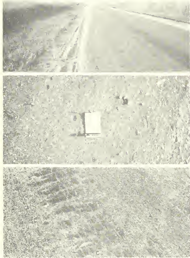
FIGURE 11.—A, CUT-BACK SECTION AFTER RE-TREATMENT. THE GRASS LINE MARKS THE EDGE OF THE ORIGINAL BITUMINOUS MAT AND THE ARROW MARKS THE EDGE OF THE RE-TREATMENT. LOOSE MATERIAL NEAR THE EDGES HAS BEEN WHIPPED TO THE SIDES BY TRAFFIC. B, APPEARANCE OF THE SURFACE IMMEDIATELY AFTER RE-TREATMENT. C, APPEARANCE OF SECTION 9A 3 YEARS AFTER SURFACE TREATMENT. THE DARK STRIP IS THE AREA BETWEEN WHEEL TRACKS AND IS SLIGHTLY RAISED.
