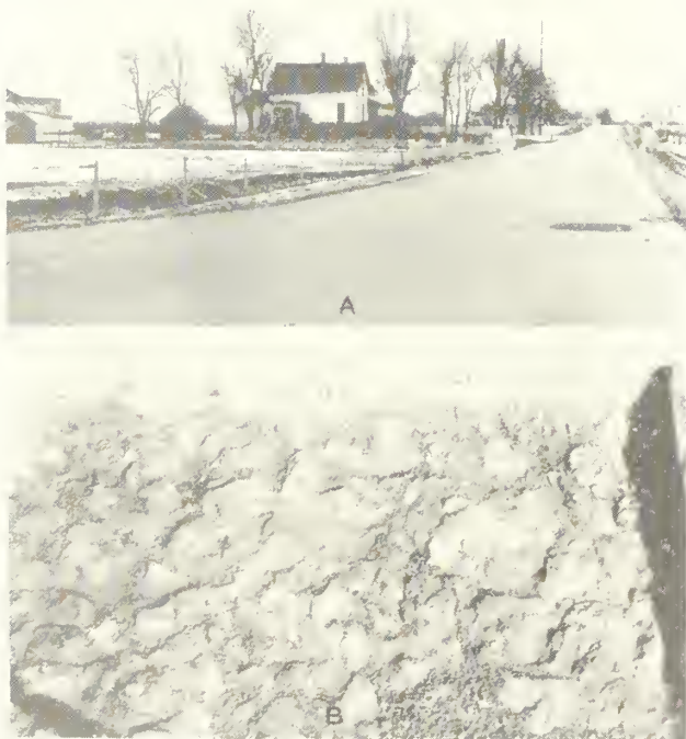
FIGURE 3. A, GENERAL VIEW OF AN EXCELLENT PAVEMENT, AND B, DETAIL OF THE GOOD WATER-BOUND MACADAM BASE EXPOSED BY REMOVAL OF THE SAMPLE. THE DARK SPOT IN THE RIGHT FOREGROUND IN A IS THE PATCH THAT WAS PLACED AFTER THE REMOVAL OF SAMPLE 11-C-1.
