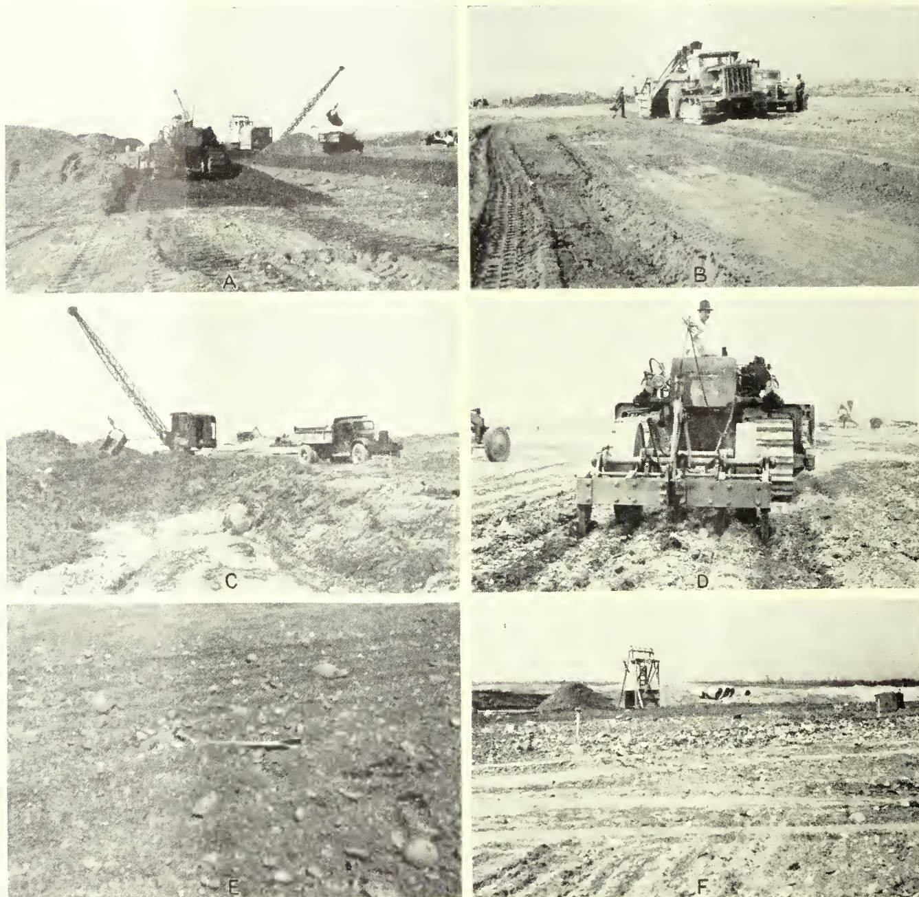
FIGURE 8.—CONSTRUCTION OF RUNWAYS: A, GRADING OPERATIONS; B, THIN LAYERS OF MUCK BEING EXCAVATED BY SCRAPER; C, DEEP MUCK BED BEING EXCAVATED BY DRAGLINE; D, SCARIFYING MATERIAL WITH HEAVY-DUTY ROOTER; E, OVERSIZE STONE BROUGHT TO SURFACE BY SCARIFYING; AND F, OVERSIZE STONE IN EXCESSIVE AMOUNTS GENERALLY ENCOUNTERED AT RUNWAY INTERSECTIONS.
