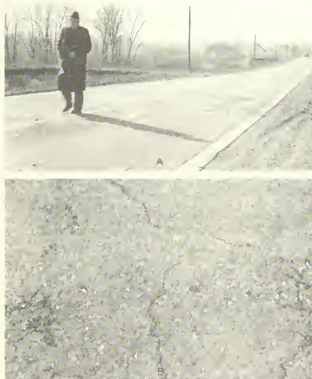
FIGURE 2.—A, GENERAL VIEW, AND B, SURFACE DETAIL OF A PAVEMENT THAT WAS RATED VERY POOR. NOTE THE SPALLING ALONG THE CRACKS AND THE RAVELED CONDITION OVER A LARGE PORTION OF THE PAVEMENT. SAMPLE 8-B WAS TAKEN AT THIS LOCATION. THE PATCHED SAMPLE HOLE CAN BE SEEN IN THE RIGHT CENTER OF THE UPPER PICTURE.
