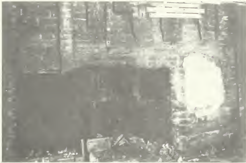
Illustration 52. Antram-Gray House: Uncovered First-Story Fireplace at North End of West Wall (Formerly in Room 204).
