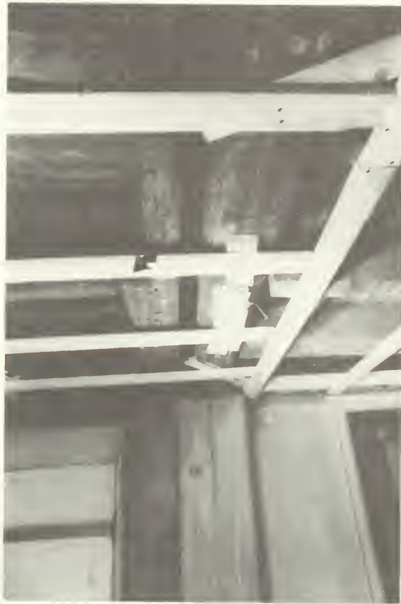
Illustration 48. Antram-Gray House: First-Floor Framing, Showing Circa-1730 South Girt Cut Out for Southeast Stair.
