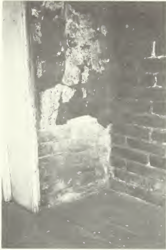
Illustration 44. Antram-Gray House: Fireplace in Room 202, East Side of Firebox, Showing Natural-Cement Targeting.
