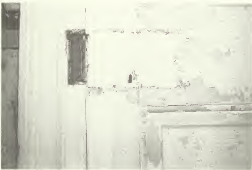
Illustration 45. Antram-Gray House: Door 204, South Side, Showing Paint Evidence of Missing Rim Lock.
