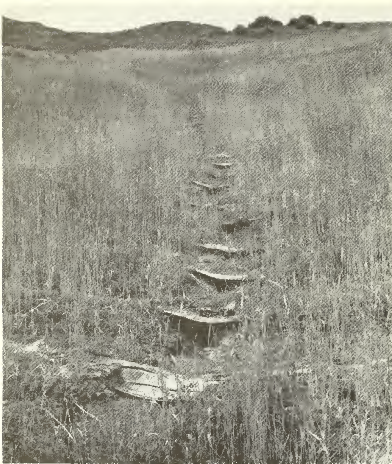
Figure 6.—Looking upstream on middle reach of Alkali Creek waterway No. 18, where V-shaped waterway cross sections caused concentrations of flow.
