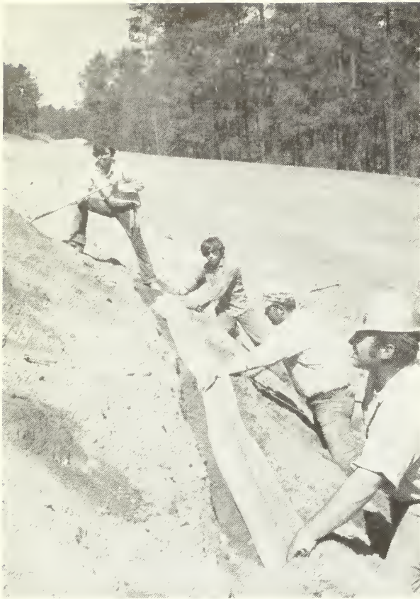
Figure 2.—Placement of burlap strip into trench of road-cut slope on the Gila National Forest.
