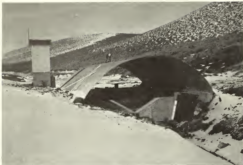
Figure 1.—A sharp-crested weir covered by a multiplate arch. The ends of the arch were later enclosed.
