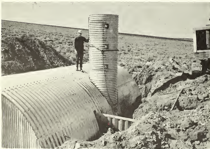
Figure 6.—A nearly completed enclosed weir showing the instrument-shelter mounting and cutoff wall placement.
