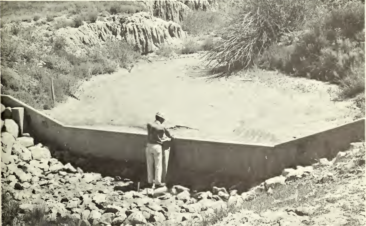
Figure 1.--After one year, sediment has collected to the crest of a prefabricated concrete check dam. Rock riprap below the dam protects gully bottom and side slopes from impact of falling water and the eddies near the banks.
