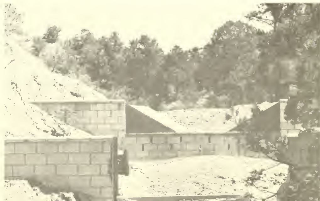
Figure 5.--A view looking upstream into the sediment basin after at least 18 tons of sediment had passed through the flume in a single flow. (The downstream sediment basin wall failed.) Flume sidewalls were scratched, but there were no dimensional changes.
