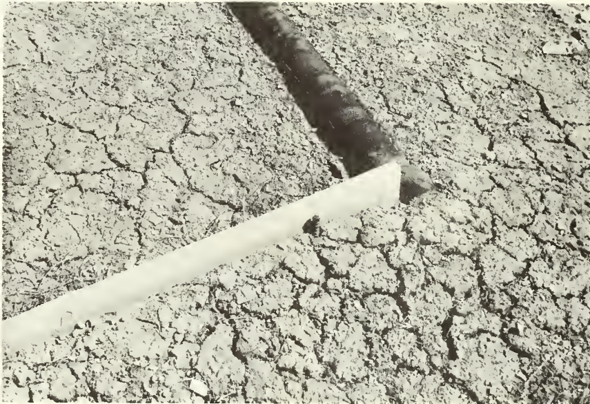
Figure 15.--Corner of plot border and collection trough 4 years after installation. No maintenance was needed.
