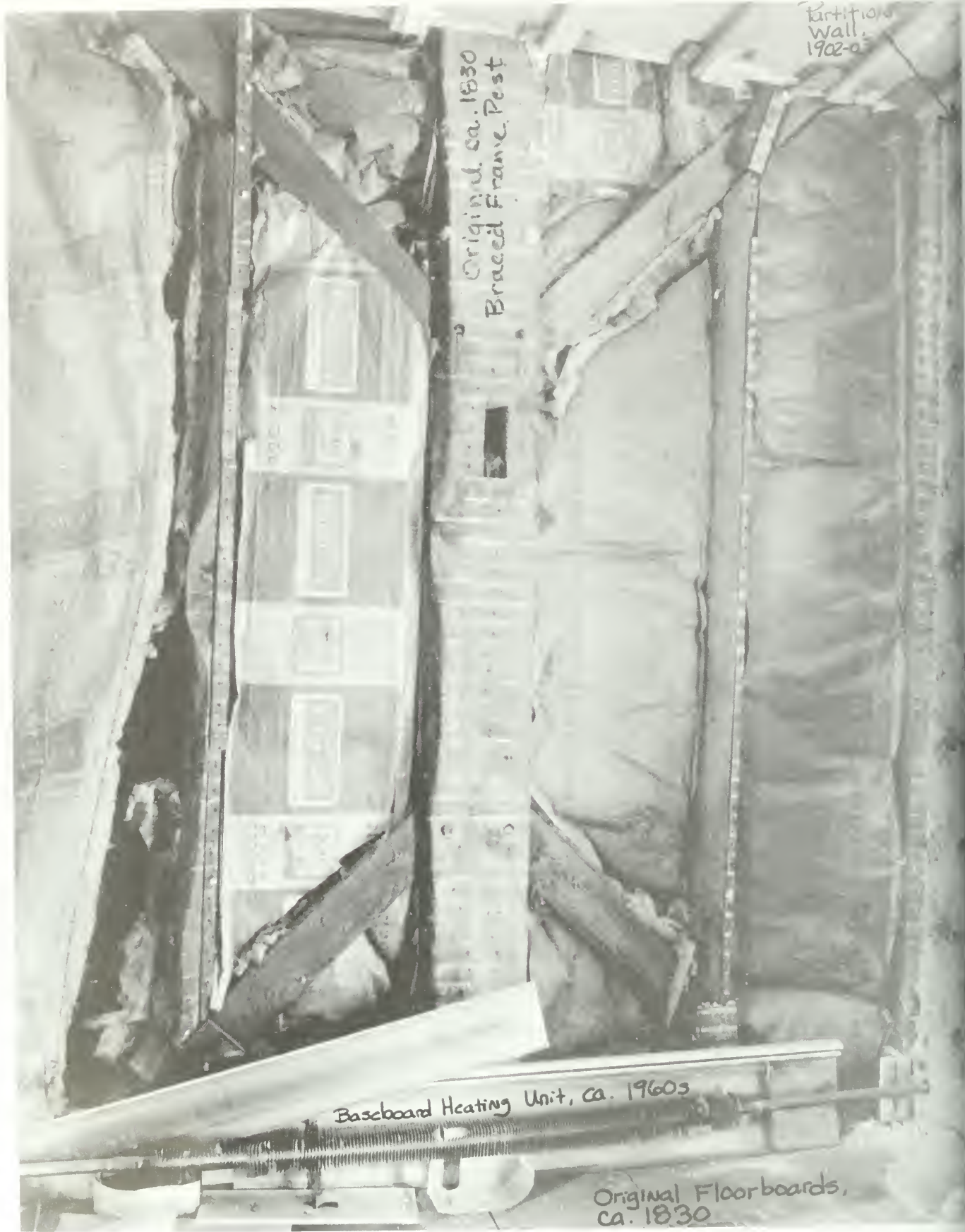
Figure 58. Stanton House: second-story hall. detail of braced-frame post at north wall, July 1982.
