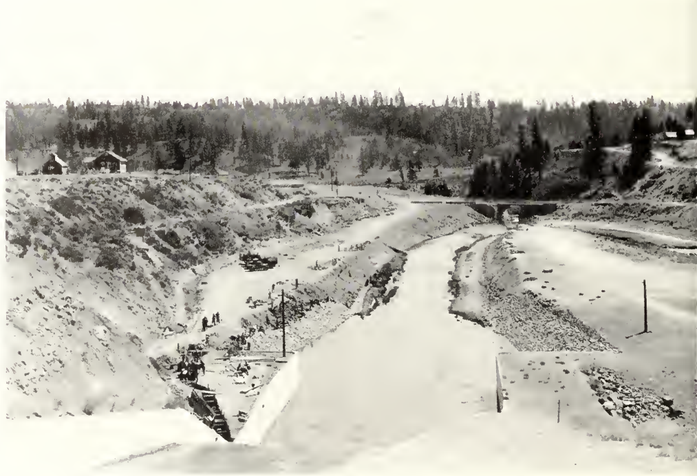
Looking down spillway outlet channel of Boca Dam. Riprap work in progress
