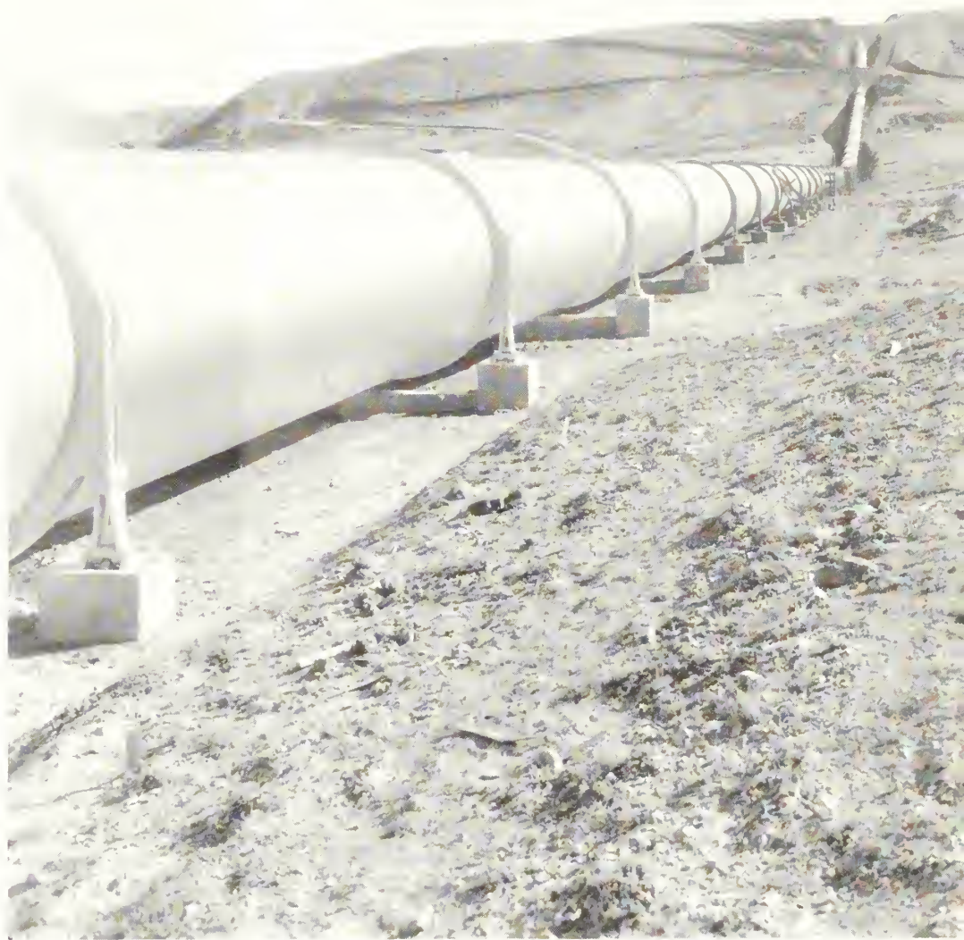
Buck Springs Creek Siphon (Shoshone project) viewed from Heart Mountain Canal Backfill operations on monolithic concrete barrel section in background.
