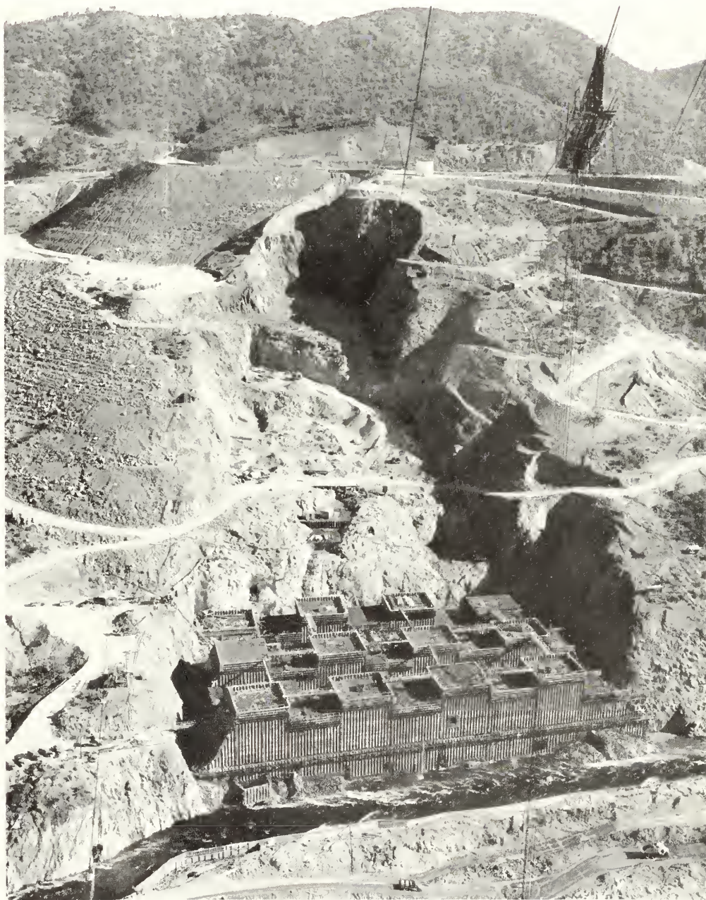
Before the close of September 1940, about 150,000 cubic yards of concrete had been placed in the left abutment of Shasta Dam
