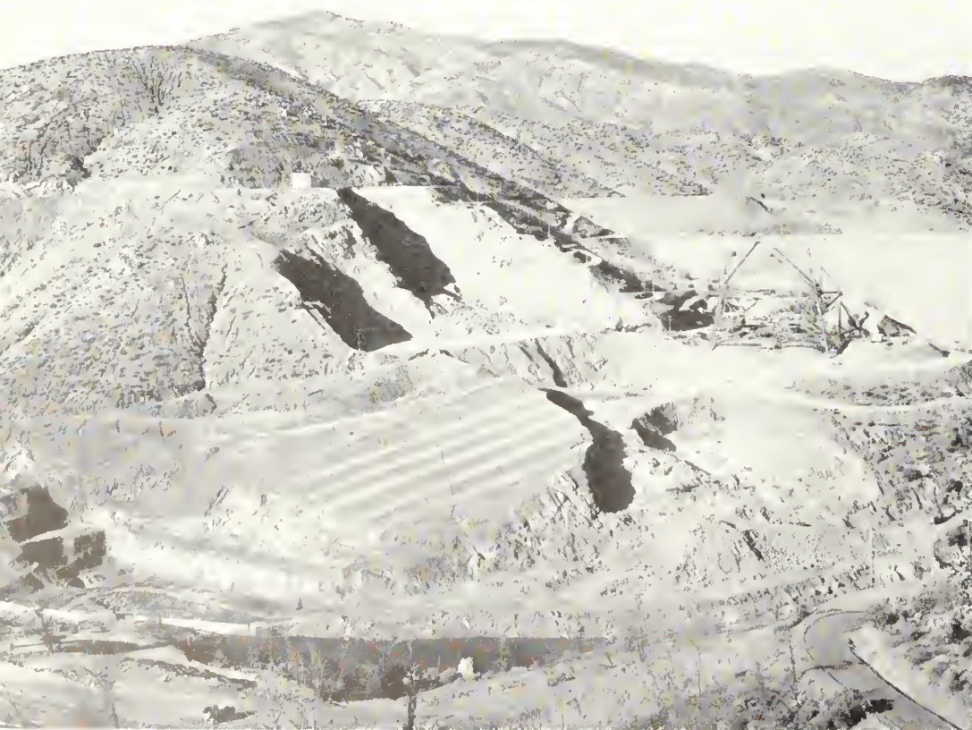
Shasta Dam from left abutment roadway, showing operations on right abutment, Powerhouse and penstock areas, abutment excavation, cableway headtower, and a portion of the stock pile area
