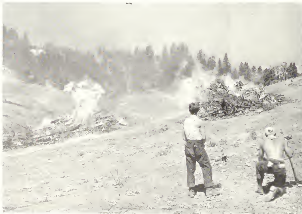
Enrollees burn the trees and brush cleared from Shasta Dam Reservoir site, Central Valley project, California
