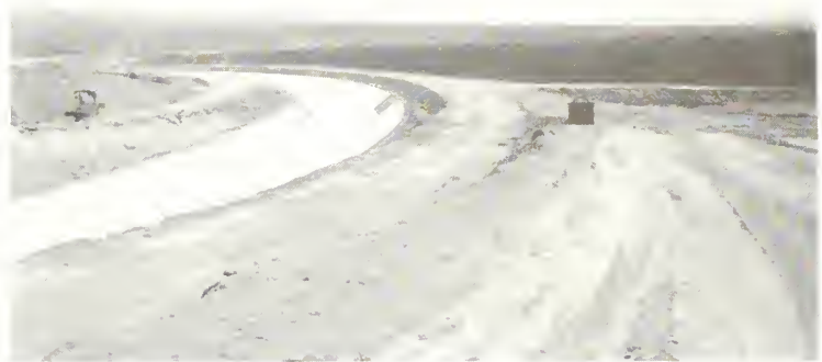
Photo 5: Lined canal. The concrete is first painted with coal-tar cut-back and then coated with whitewash as a temperature control. The dark patches on the lining are openings left for the piers of a bridge to be constructed.
