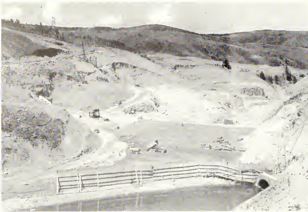
Cofferdam, with diversion dam and tunnel in foreground; main dam foundation in central background
