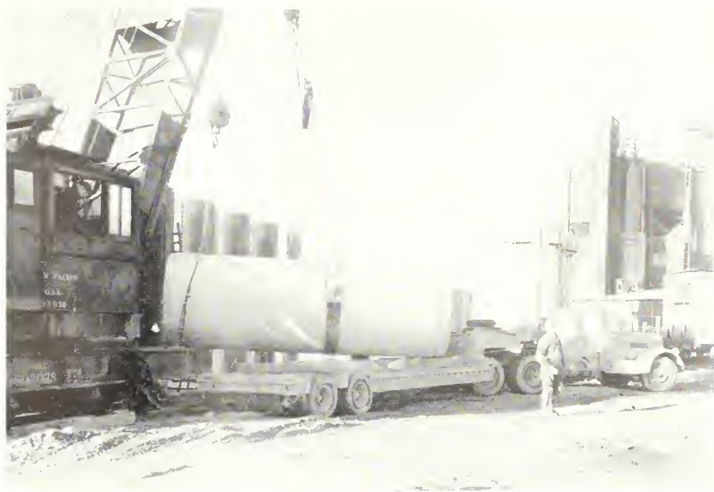
Twenty-foot section of test pipe, weighing 20 tons, being loaded onto special trailer
