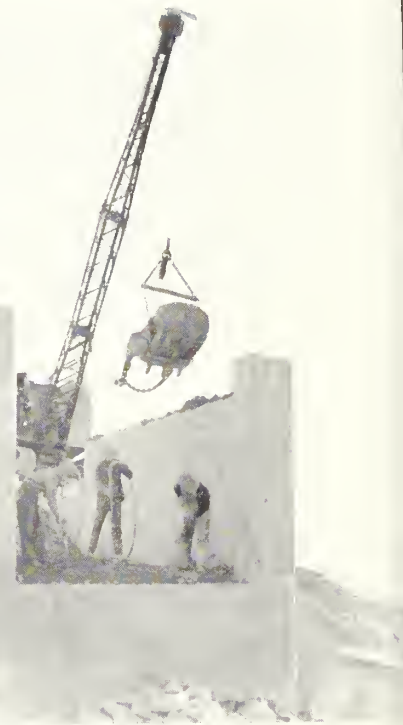
Concrete bent and abutment for steel supporting 72-inch diameter steel pipe span used over natural drainage channel
