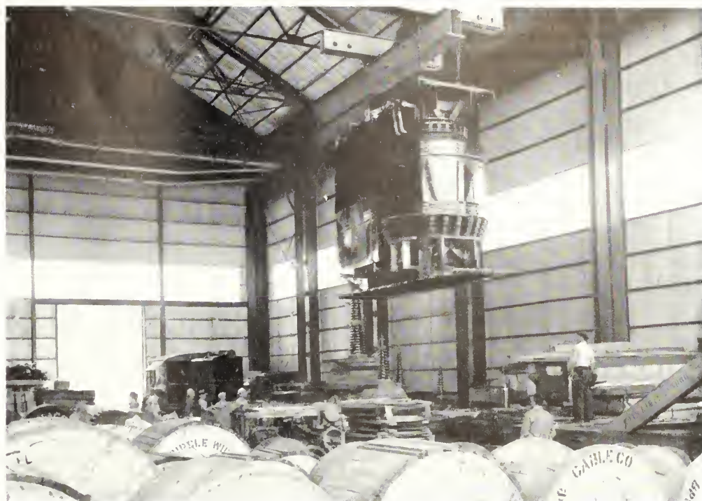
Eighty-ton core and coil for 55,000-kilovolt-ampere single-phase transformer after being removed from transformer car tank
