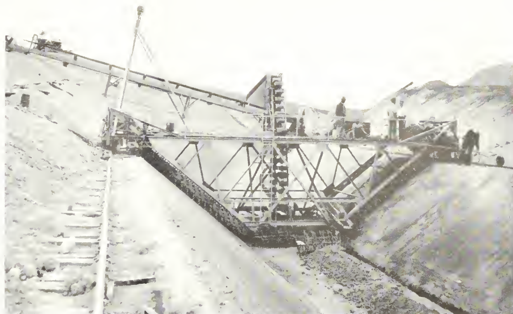
Photo 1: Trimming machine. Note rotating drum teeth, trimming arrangement, and screw-carrying device in canal invert.
