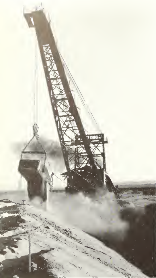
Above: 16-cubic-yard bucket of Monighan walking dragline dumping load on canal embankment
