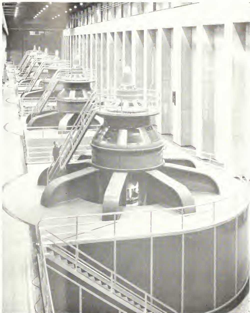
Six 82,500 kilovolt-ampere generators, biggest in the world, in the Nevada wing of the powerhouse at Boulder Dam, with one in the Arizona wing, produce power amounting to 130,000,000 kilowatt-hours of energy each month which sells for $290,000
