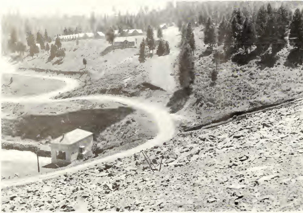
Needle-valve house, downstream slope of Boca Dam at west abutment, and CCC camp. Road construction and drainage installations partially completed
