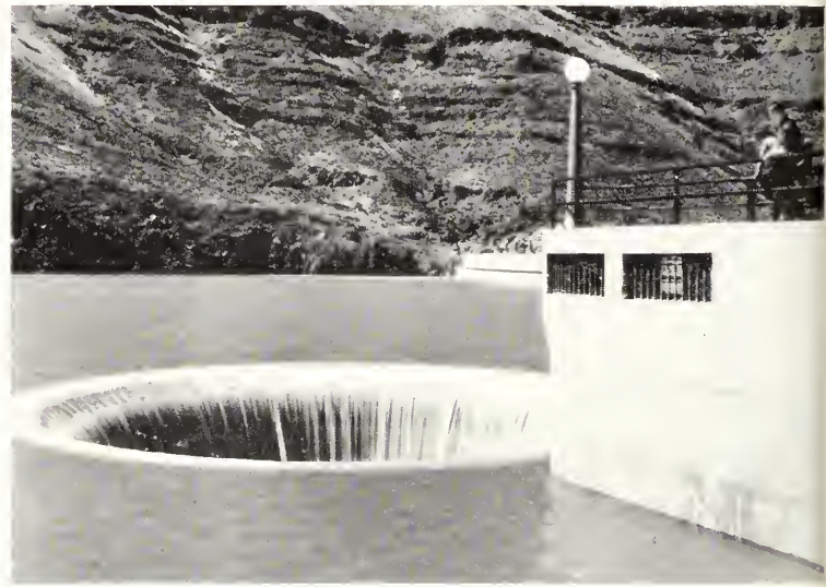
Figure 10. Spillway discharging a very thin film of water over ring gate crest. The radially converging flow is plainly seen here.
