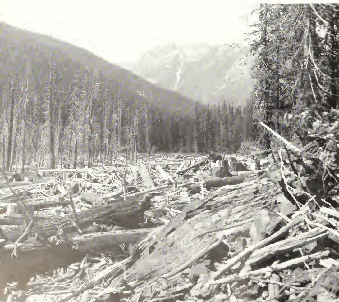
Upper end of Lake Kachess before beginning the clearing operations by CCC enrollees
