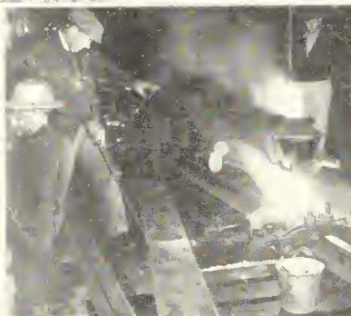
A "Thermit" pressure weld on a 131-lb. rail joint of the relocated railroad around Shasta reservoir site, California
