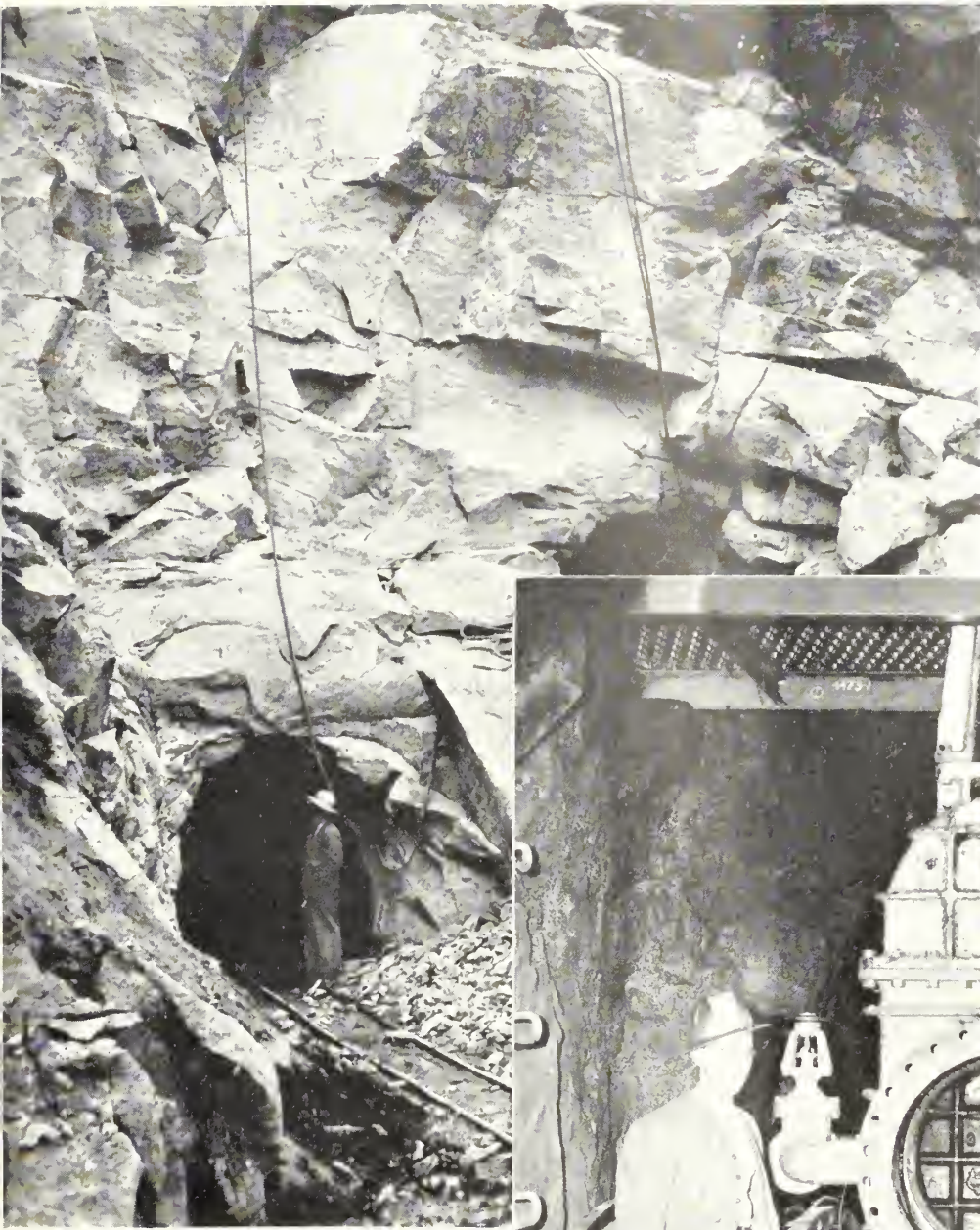
Lower portal, Snow Lake main tunnel, tapping upper Snow Lake, and adit tunnel to control gate chamber
