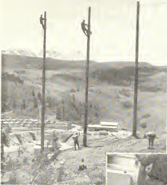
TRANSMISSION LINE at Green Mountain Dam site Colorado.
