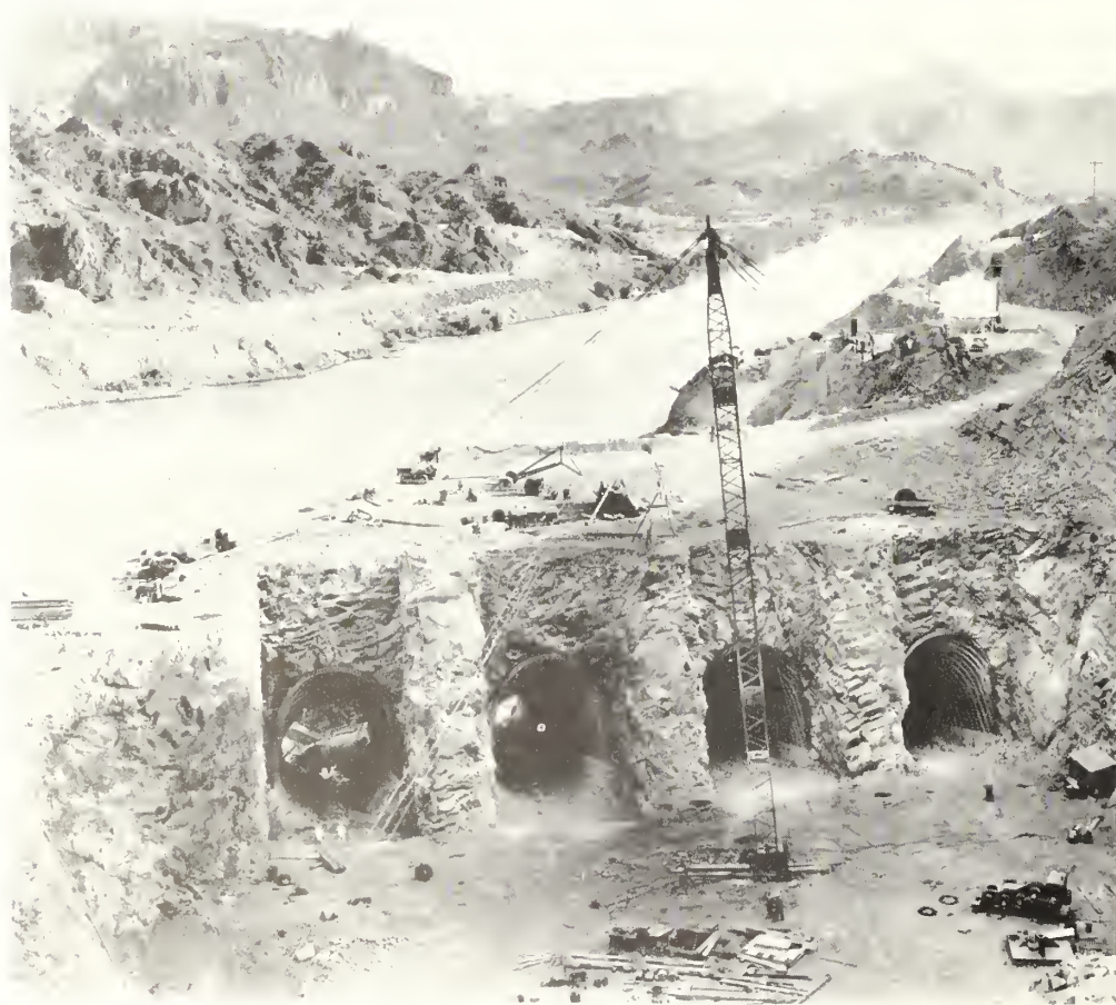
Inlets to four 27-foot diameter penstock tunnels. Flared transitions at the upstream end of each tunnel result in an opening 27 feet wide by 40 feet high
