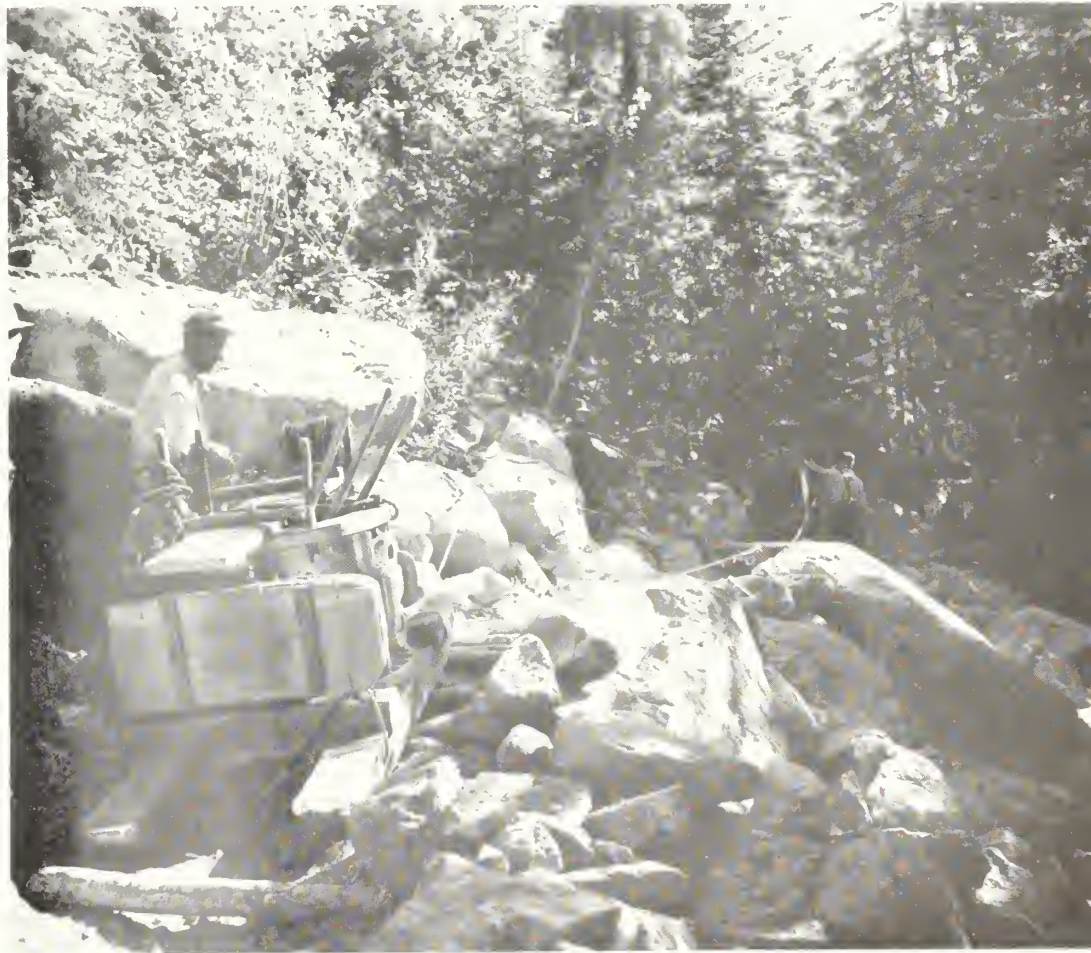
Conveying a heavy valve over a rocky trail in the Cascade Mountains for the control of the flow of cold water from a high mountain lake to an enormous fish hatchery under construction at Leavenworth, Wash.
