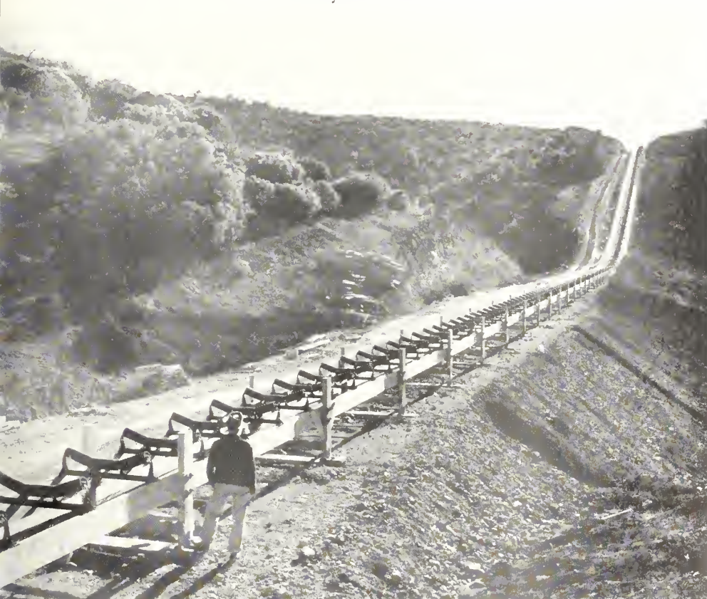
Section of aggregate conveyor under construction, showing trough rollers in place ready for belt
