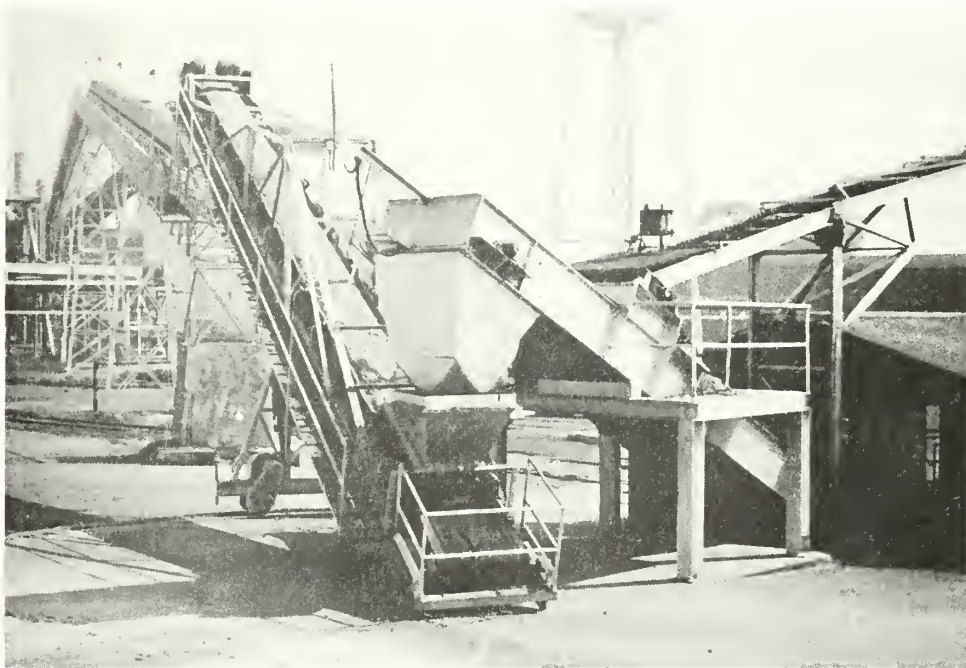
Chip handling by conveyors, from pit to movable transfer section, then either to plant as shown or to storage piles.
