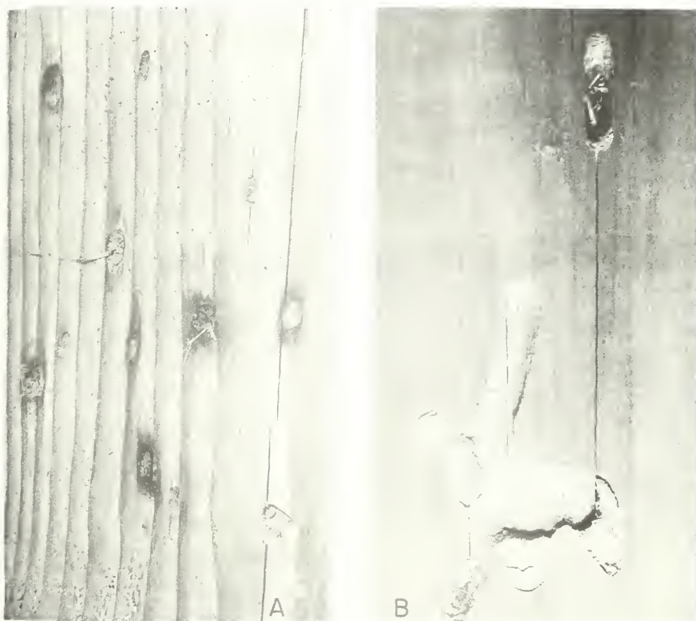
Figure 3. Larval tunnels packed with borings in Douglas-fir. A , board with several tunnels in cross section (Photo courtesy R. D. Hodges); B , longitudinal section through part of tunnels.
