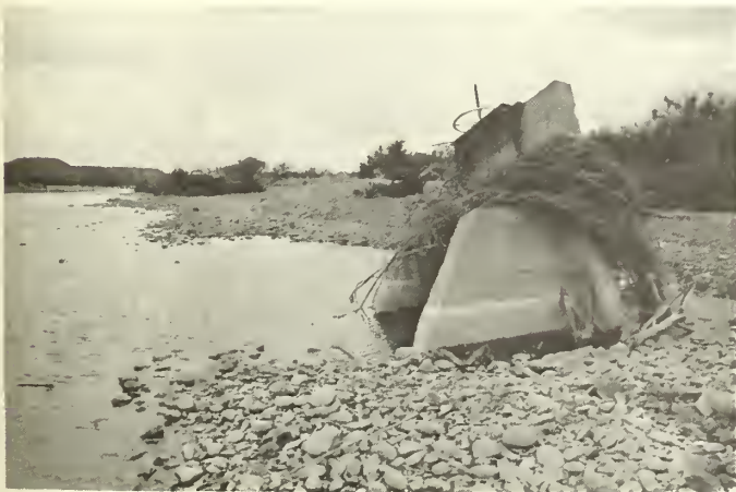
Figure 3.—High stagnation pressures from shooting flows of the unusual January 1979 flood in the Verde River, central Arizona, created uplift forces that aided in upsetting this water-diversion structure and a 2-foot-diameter concrete pipeline.
