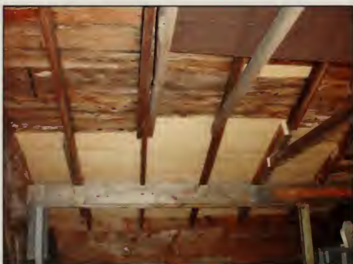
Figure 273. Ceiling of Room 101, Garage. Note sheathing repairs, placement of beam to support rafters, and sistering of collar ties between rafters (2007).
