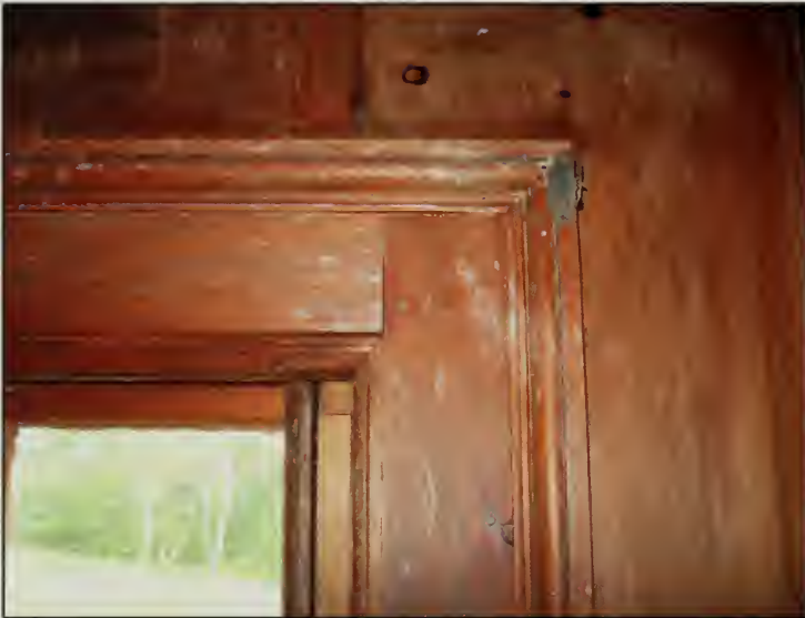
Figure 412. Example of interior window trim surrounding windows in South Bedroom, Guest House (2007).
