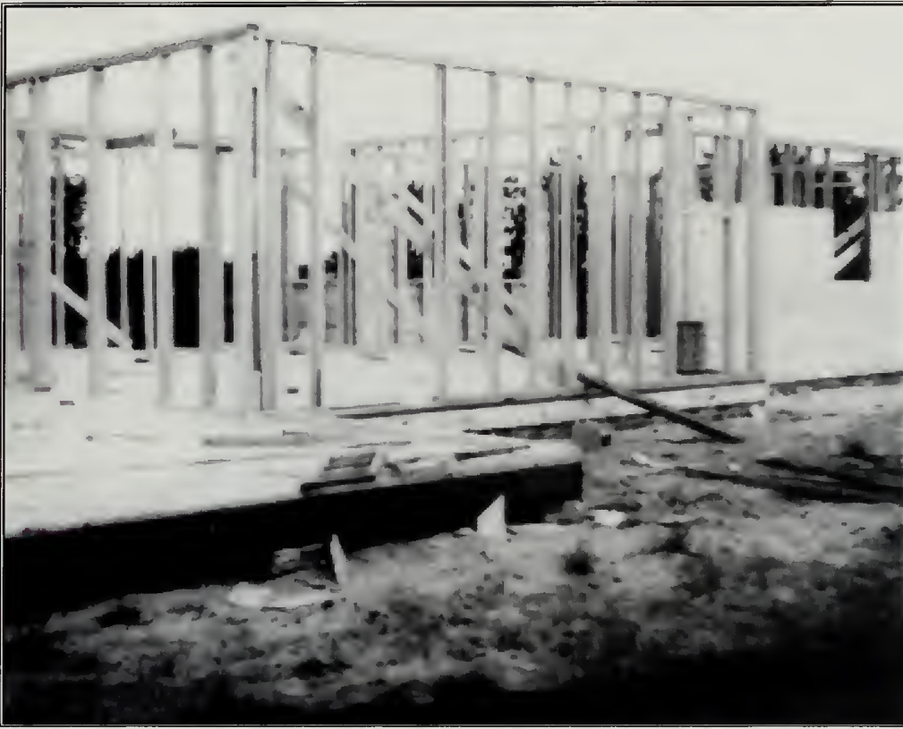
Figure 224. Photograph of construction framing of the west elevation of the Country Store in 1947. (GKH Journal, p. 112).
