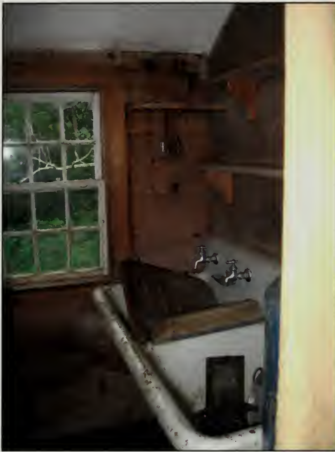
Figure 249. East and south wall shelving and white porcelain sink on south wall in Laundry section of Laundry/Bath addition, Woodshed (2007).
