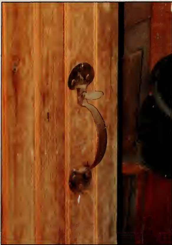
Figure 245. Thumb latch on the door between Storage Room and Laundry section of Laundry/Bath addition, Woodshed (2007).
