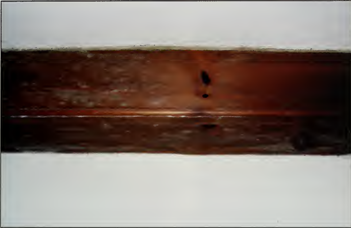
Figure 408. Example of cased girts and beams of the structural framing system exposed on all walls in the South Bedroom, Guest House (2007).
