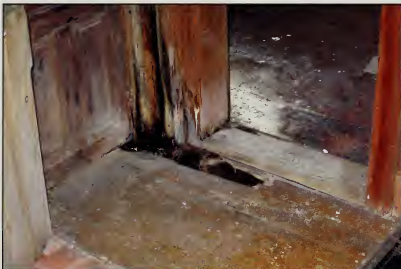
Figure 390. Large hole in northeast corner of floor in Living Room, Guest House (2007).
