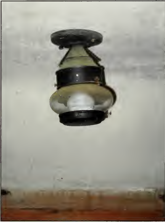
Figure 247. Light fixture in Laundry section of Laundry/Bath addition, Woodshed (2007).
