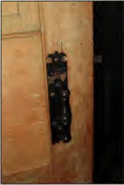
Figure 411. Iron thumb latch on door within D109 in South Bedroom, Guest House (2007).
