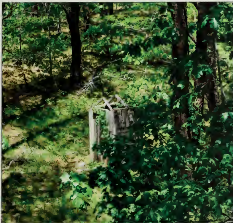
Figure 87. Privy in poor condition, without a roof, set off in the woods northwest of the Country Store. (OCLP, May 2010.)
