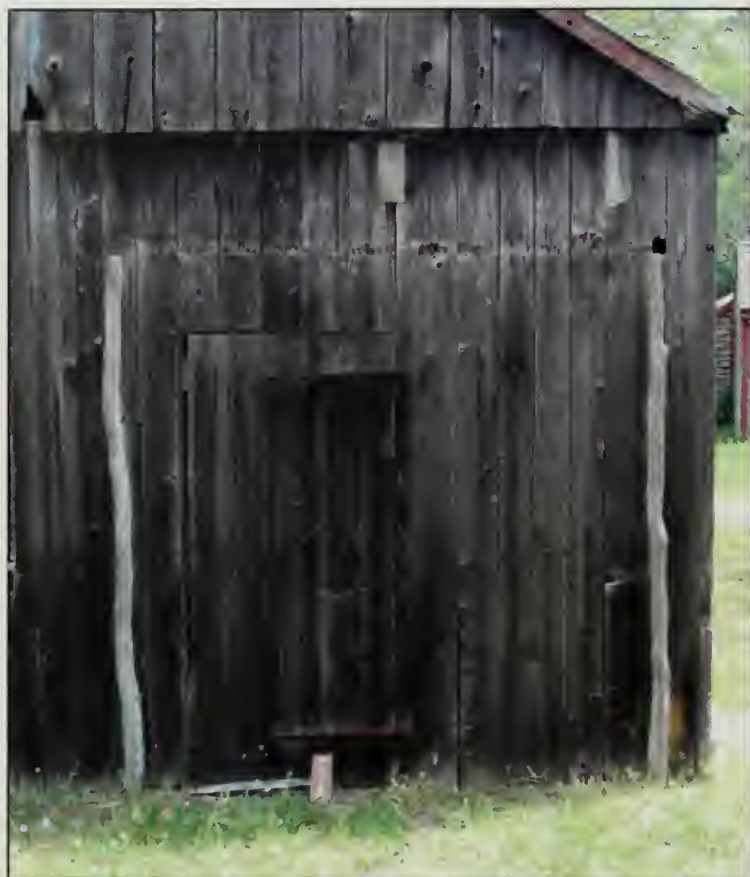
Figure 306. Wooden posts that once supported a former open porch roof, west elevation, Barn (2007).
