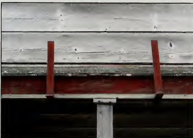
Figure 503. Two metal brackets affixed to center of the porch roof on east elevation, Country Store (2007).
