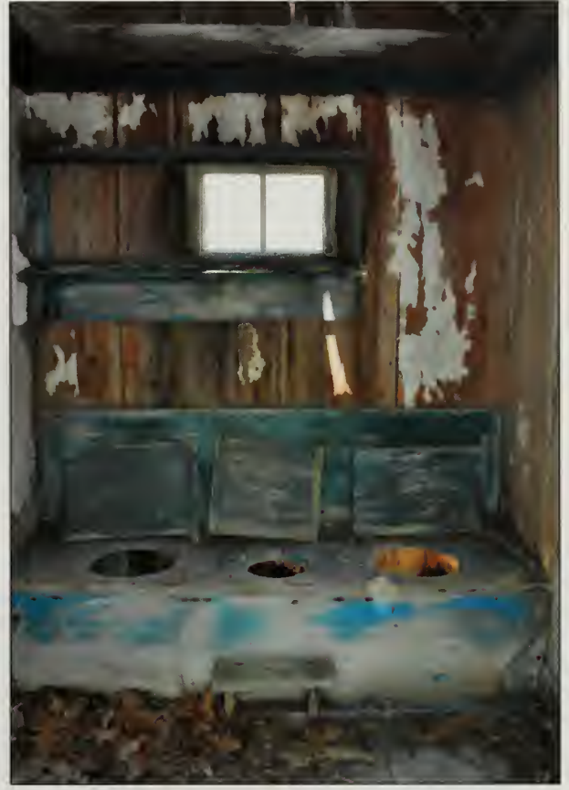
Figure 540. Interior view of north wall and seats in Guest House Privy (OCLP, August 2010).
