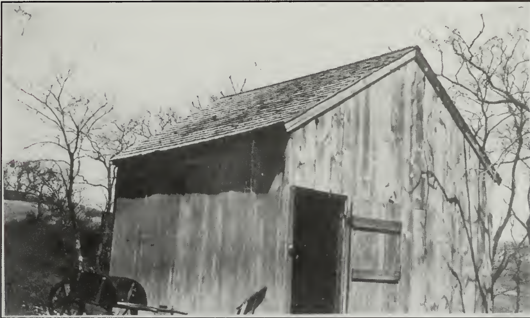
Figure 201. Woodshed, northeast of the main Atwood-Higgins house, as it appeared in 1919 when George K. Higgins acquired the Atwood-Higgins property. Note flush vertical wooden 'slab-sided' exterior walls. (GKH Journal, p. 35).
