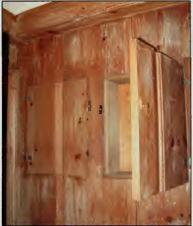
Figure 415. Two built-in cabinets on west end of north wall in South Bedroom, Guest House (2007).
