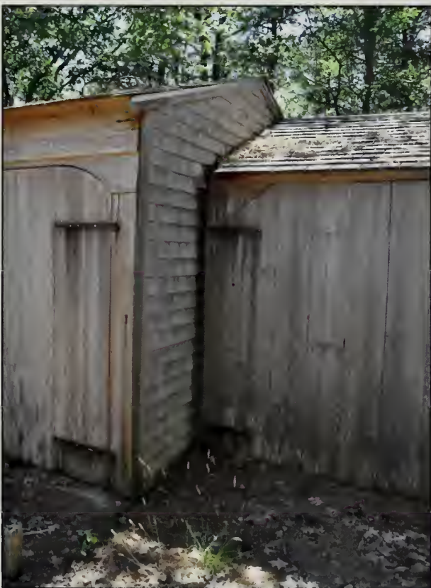
Figure 264. Detail of northeast elevation where exterior of Room 101 joins with exterior of Room 102. Note curved top corner of D102 and the cut top corner of D103 (OCLP, 2010).
