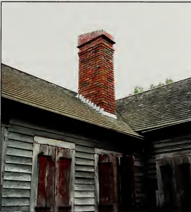
Figure 502. Chimney on east slope of the north-south gable roof over the Study, Country Store (2007).
