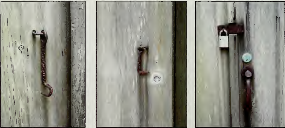
Figure 261. Hardware on door within D 101: large hook and eye fastener, small hook and eye fastener, modern embedded deadbolt, modern padlock, and iron thumb latch door pull. Northeast elevation, Garage (2007).
