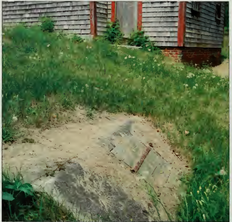
Figure 78. Concrete tank associated with drainage system, described as a cistern and as a dry well, with wooden cover by Woodshed, looking north. (OCLP, July 2007.)
