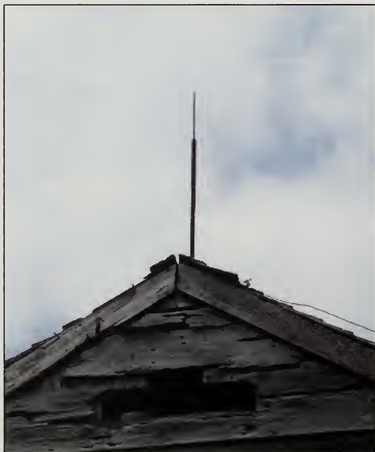
Figure 307. Lightning rod on eastern end of gable roof, Barn (2007).
