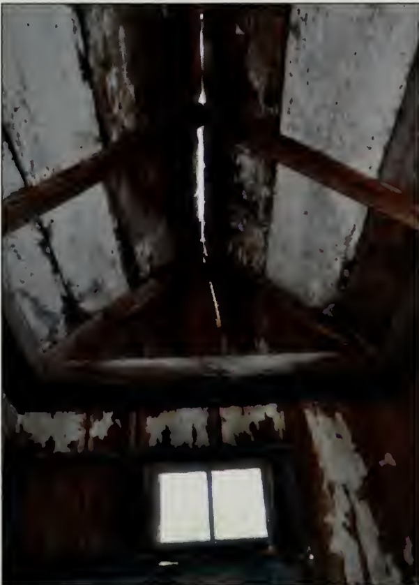
Figure 541. Interior view of north wall and ceiling, Guest House Privy (OCLP, August 2010).
