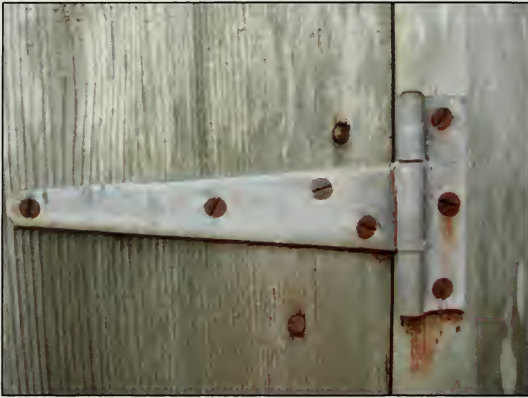
Figure 459. Metal strap hinge on door within D101 in east elevation, Summer House (2007).
