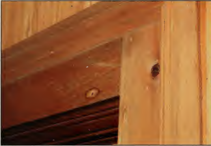
Figure 435. Window trim on W108 iof Closet, Guest House (2007).
