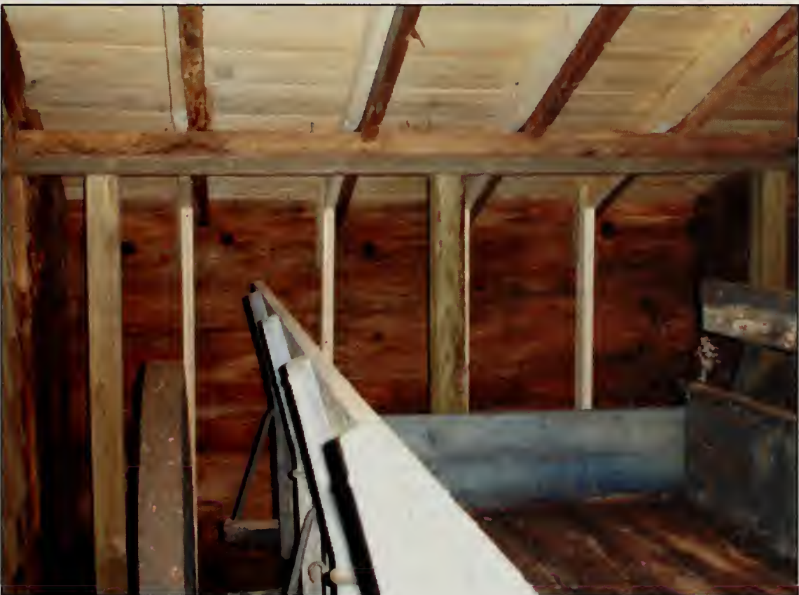
Figure 280. Ceiling and wall, southwest elevation, of Room 102, Garage. Note replaced sheathing boards, sistered rafters, sistered rafter support beam, and support posts (2007).
