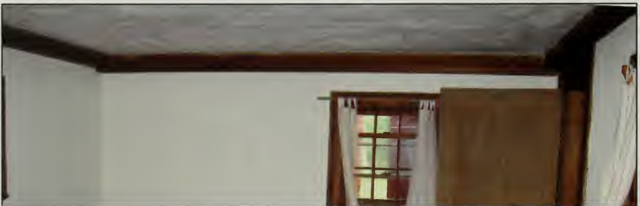
Figure 431. Ceiling and exposed beams and girts of the framing system of North Bedroom, Guest House (2007).
