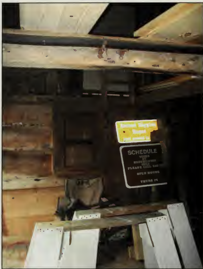
Figure 243. Built-in cabinet and wall ladder, north wall in the Storage Room, Woodshed (2007).
