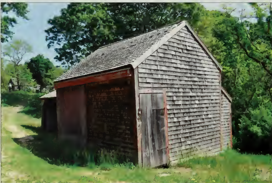
Figure 143. Looking northeast toward the Woodshed and the hillside beyond. Note the loss of the trellis structure. The vine remains but is small, May 2010. (OCLP)
