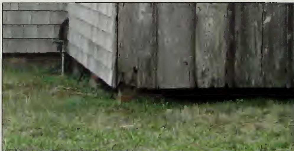
Figure 476. Brick pier foundation under north projection (Store Room and Bath), Country Store (2007).
