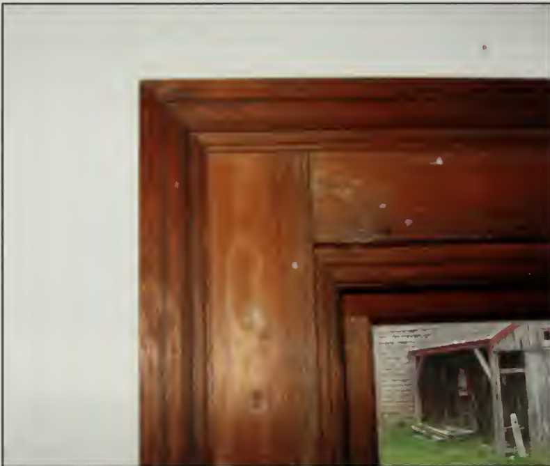
Figure 430. Example of interior window trim on windows in North Bedroom, Guest House (2007).
