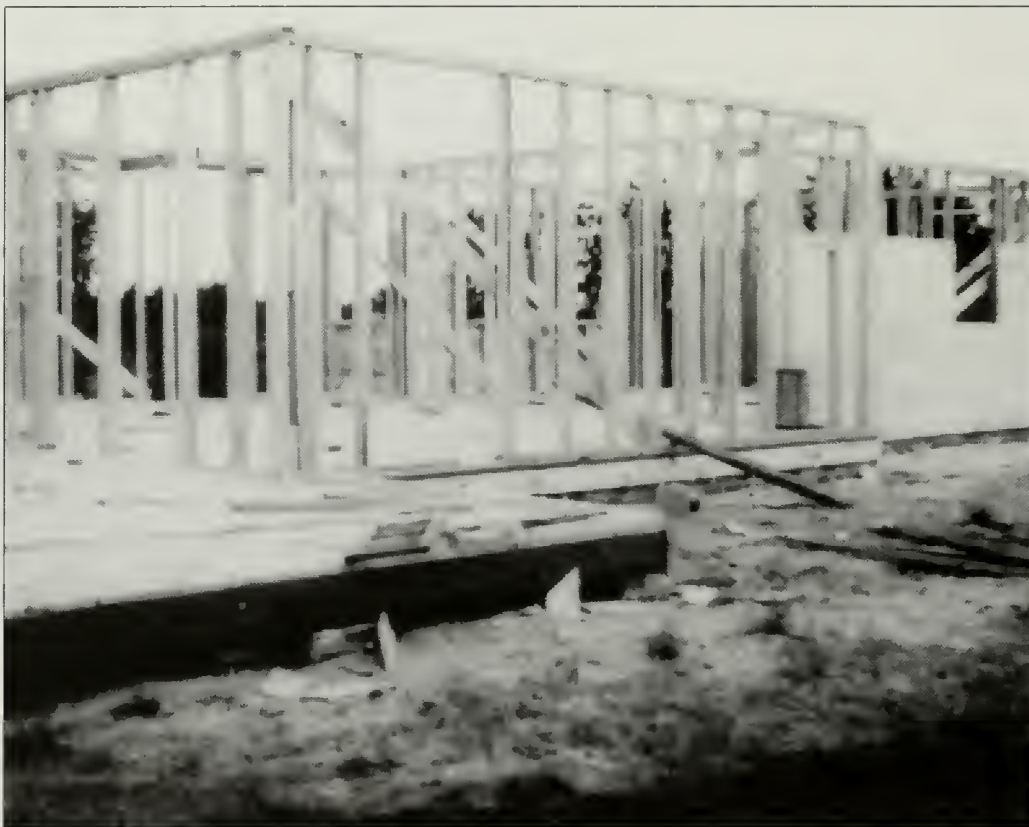
Figure 26. Country Store being built, most likely as seen looking southeast from the driveway, in 1947. (Cape Cod NS archives, H6-097.)
