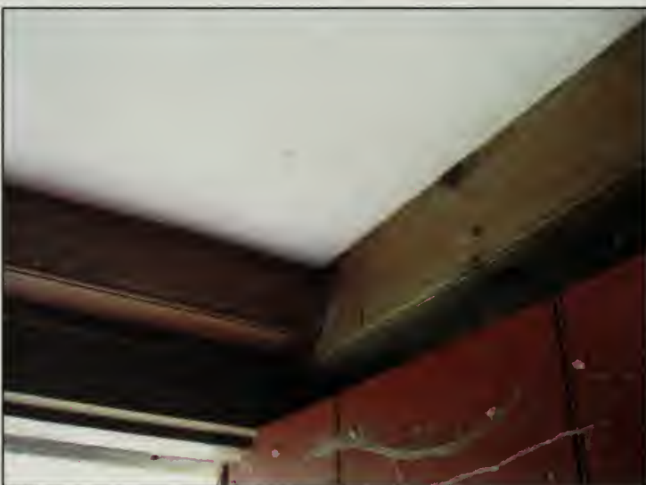
Figure 413. Example of exposed beams and girts cased with beaded boards of the post and girt framing seen on the perimeters of the ceiling in South Bedroom, Guest House (2007).
