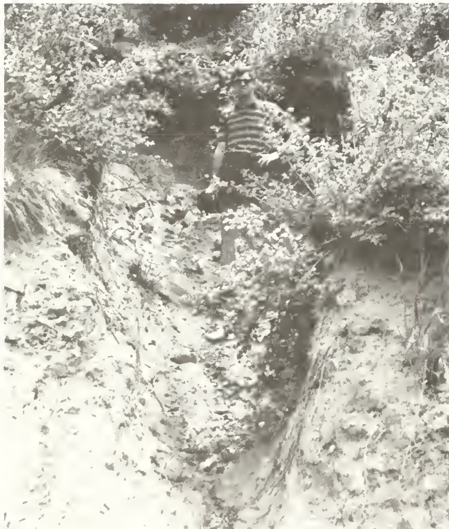
Figure 11. — Large gully in slope, Watershed No. 1, Pine Creek study area, Boise National Forest, Idaho. Gully was formed by subsurface flow emerging at cut face followed by piping and "spring sapping," which triggered localized slope failure. (Photo taken July 1977.)
