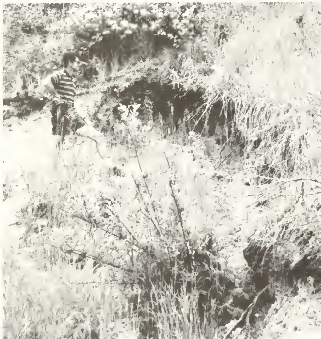
Figure 10. — Slipout in slope above road cut, Watershed No. 1, Pine Creek study area, Boise National Forest, Idaho. (Photo taken July 1977.)
