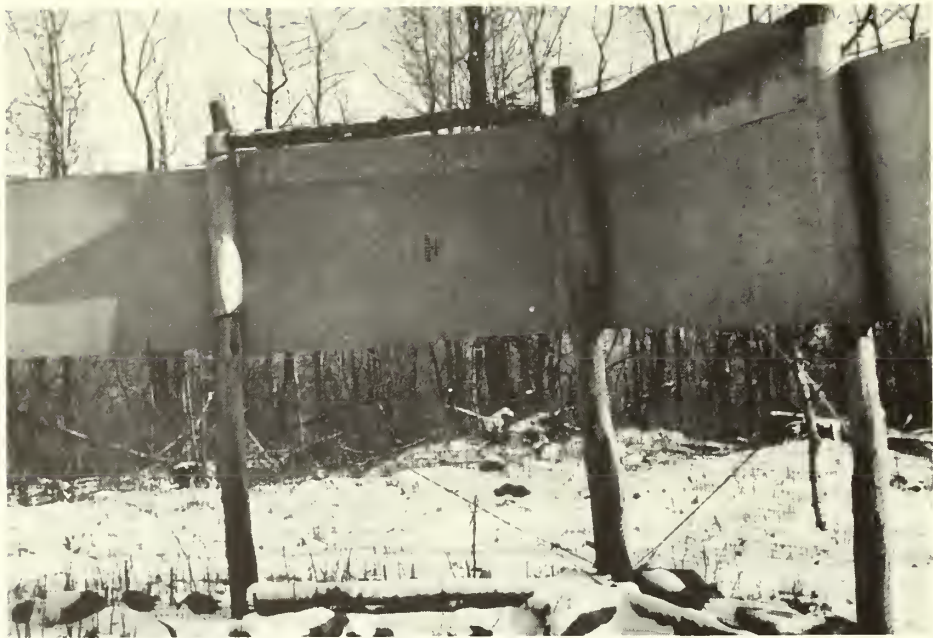
Figure 3. — Completed corner of squirrel-proof fence. Note the metal shields under the wooden braces and the wire cross bracing below the 3-foot-wide sheet metal.
