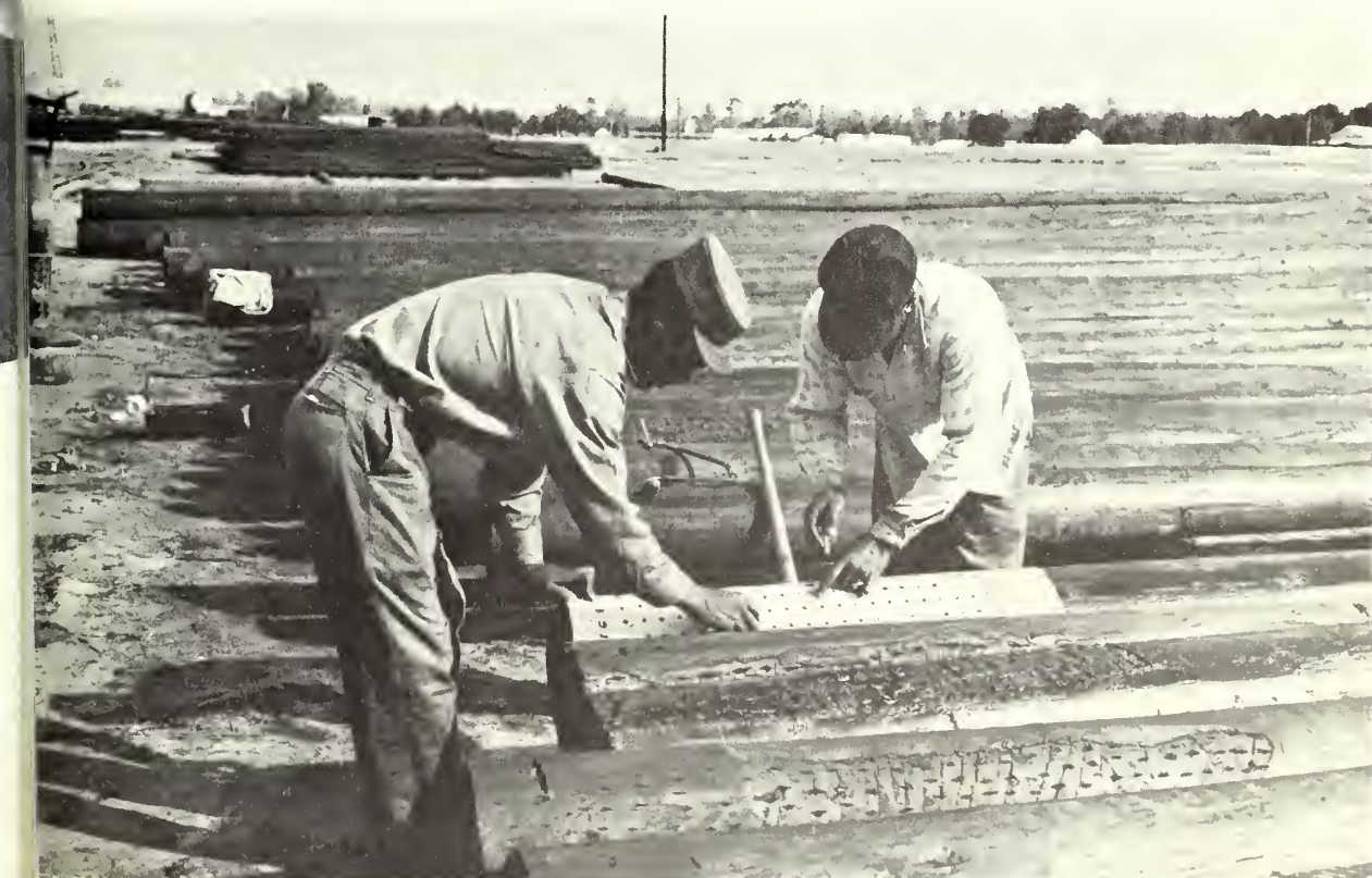
Figure 10. --Taking cores from treated poles to sample retention and penetration of preservative. Seven randomly selected test cores were taken from the turpentine-face location of all Lot I, II, III, and IV poles. An oilcloth with numbered circular holes was used to mark the location of the test cores.
