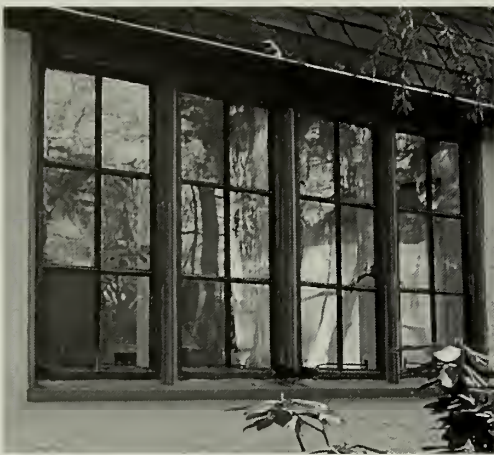
Figure 2. Each casement sash had six lights with projecting hinges that allowed the unit to open outward. Note the variation among glass panes as seen in the reflections. Caused by small differences in the positioning of panes within the sash and minor imperfections in the glass itself, this appearance is an important characteristic of historic windows.
