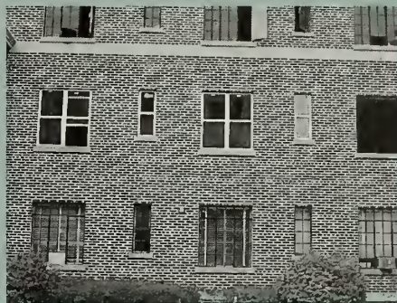
Historic steel casement windows are in the process of being replaced with new units that compromise the character of this building facade.
