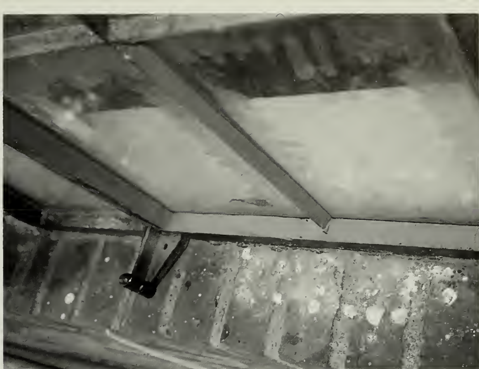
Figure 9. An oil-based putty was used to reglaze the historic casement windows. Painting was undertaken two weeks after reglazing.
