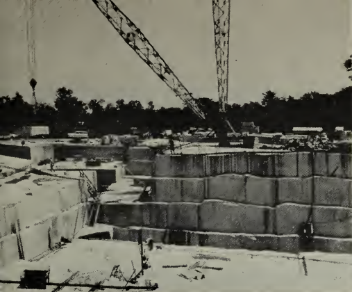
Typical bench quarry in Piedmont North Carolina from which excellent dimension granite is produced.
