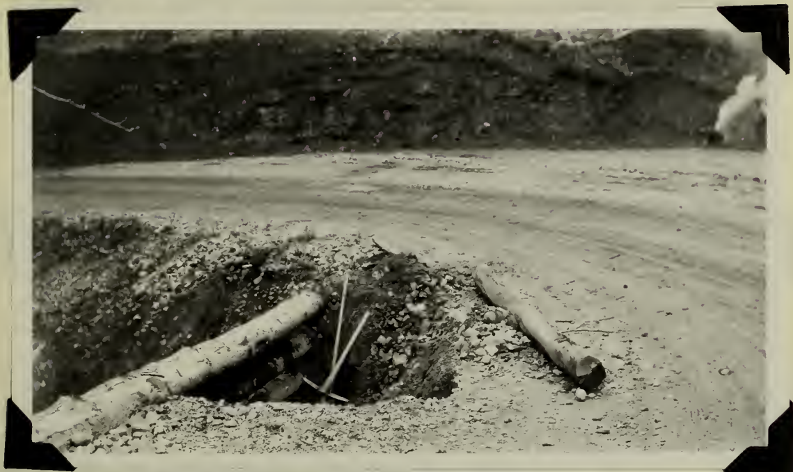
Washout, Tower Falls Road, July 10, 1930. (Partly repaired)
