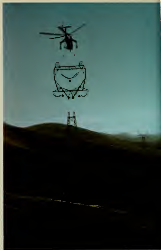
(Top) Sky Crane positions tower bridge; (Bottom) Lowering a section of transmission tower; (Right) Loading concrete for aerial delivery.
