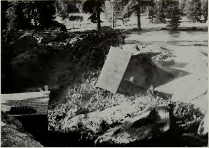
Fig. 5. Cascade Lake Dam in the initial stages of failure.
