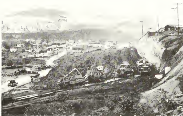
ALL ROADS LEAD TO GRAND COULEE —and the Bureau is building a four-lane highway between Grand Coulee and the top of Grand Coulee Dam. The 1.3-mile strip will use much of the existing road bed. Contractor for the paving job is Goodfellow Bros., Inc., Wenatchee, Wash.
