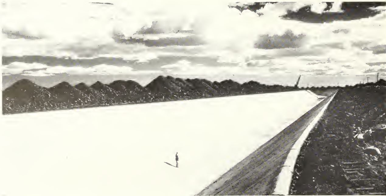
MAIN ARTERY for Irrigation Block 40 in Grant County, Washington, is East Low Canal, above. Photo by H. E. Foss, Region 1.
