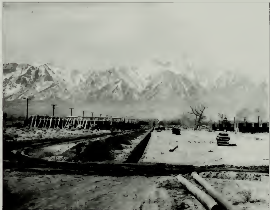
Figure 13. Water lines being installed along the camp roads as the barracks buildings are being constructed, March 1942. (Courtesy UCLA Special Collections)
