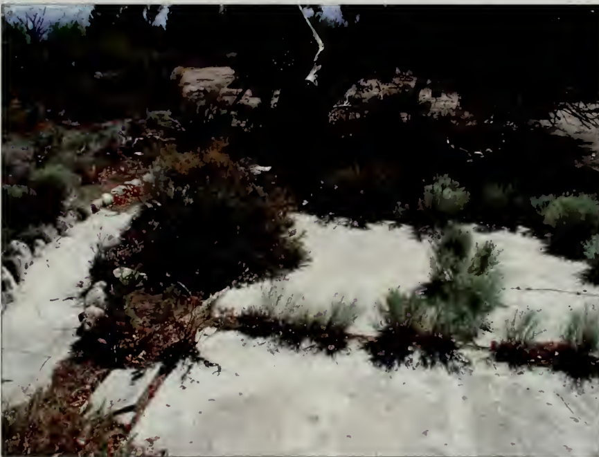
Figure 100. Non-historic vegetation obscures the historic foundations and can damage garden features if left unmanaged. (NPS, 2002)
