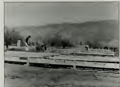
Figure 15. Contractors Griffith and Company of Los Angeles began the construction of buildings in March 1942, erecting barrack buildings at a rate of up to two buildings in one hour. (Courtesy UCLA Special Collections)
